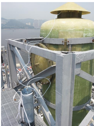
Final air scrubber
