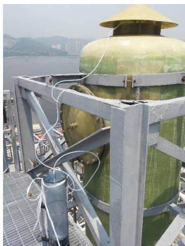
Final air scrubber
