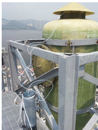
Final air scrubber
