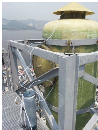
Final air scrubber
