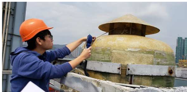
Final air scrubber
