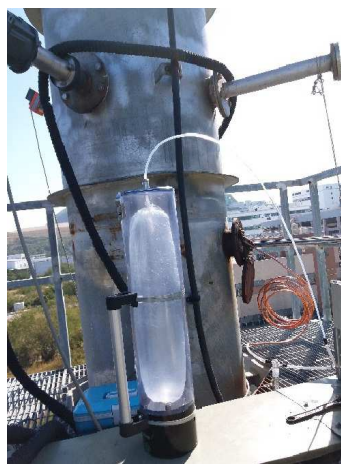
Boiler stack (EP2)
