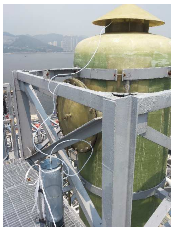
Final air scrubber
