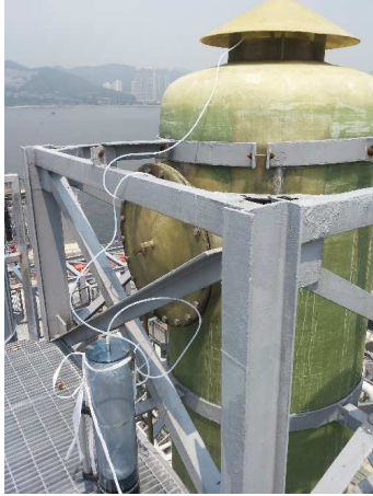
Final air scrubber
