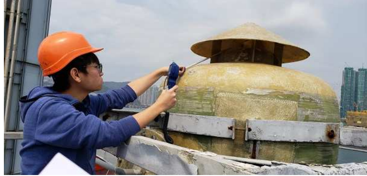
Final air scrubber
