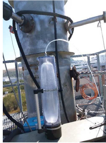
Boiler stack (EP2)
