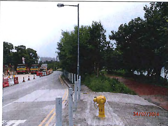
General view of works area G at southern bound of Lung Mun Road
