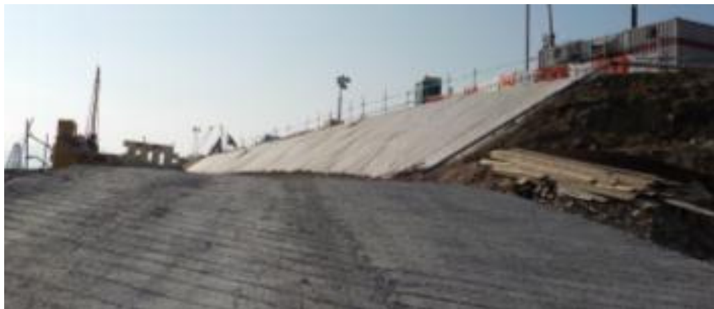
Hydroseeding and access roads paved as soon as practicable after works have been completed on soil exposed area. (Reclamation Works Area)
