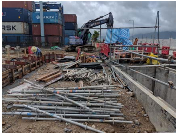
Photo 1&2 - Pump Sump Area
