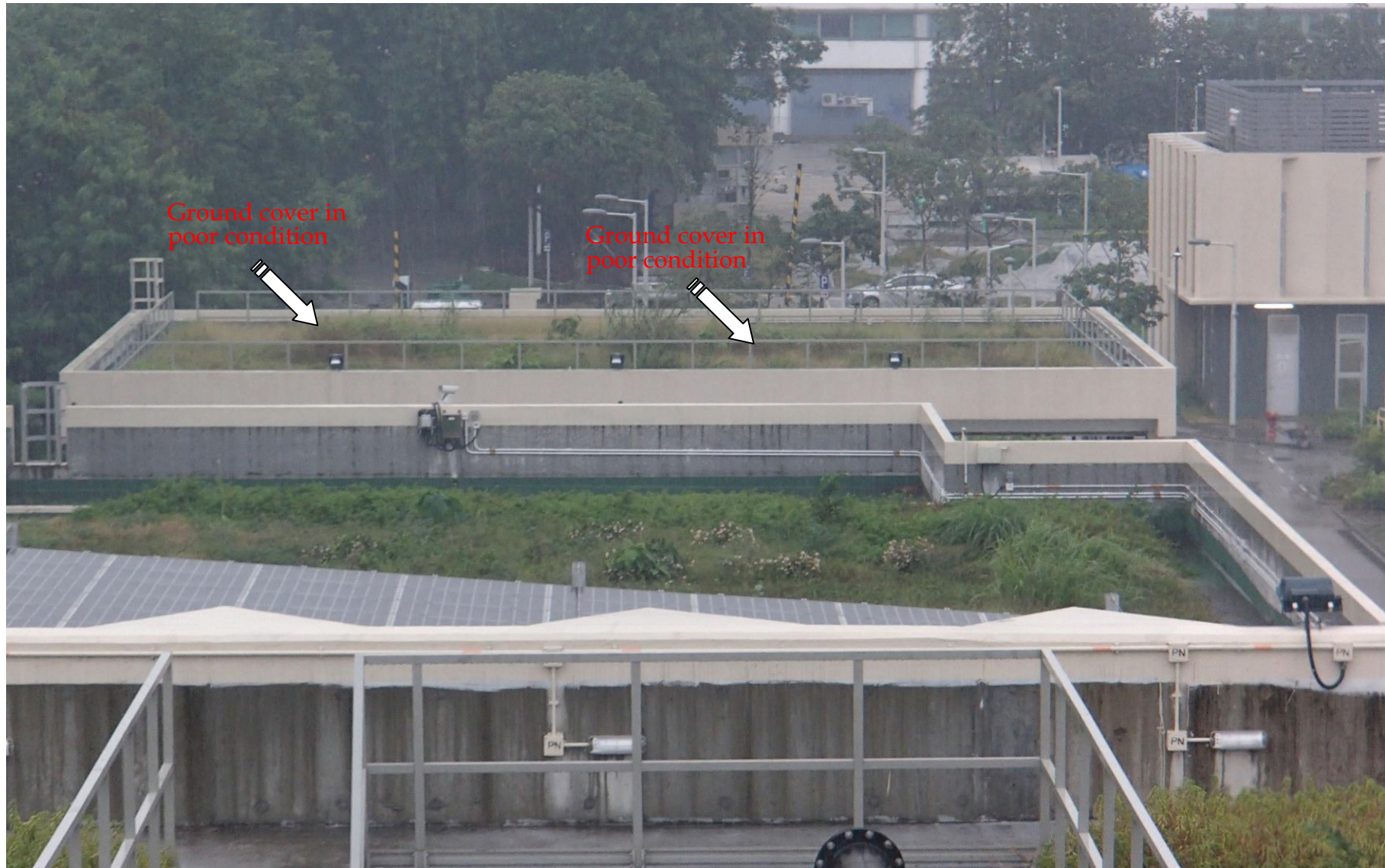
Photo no. F-03 : Groundcover & Lawn in roof garden ( Septic Waste Reception Station ) were observed in poor condition.
