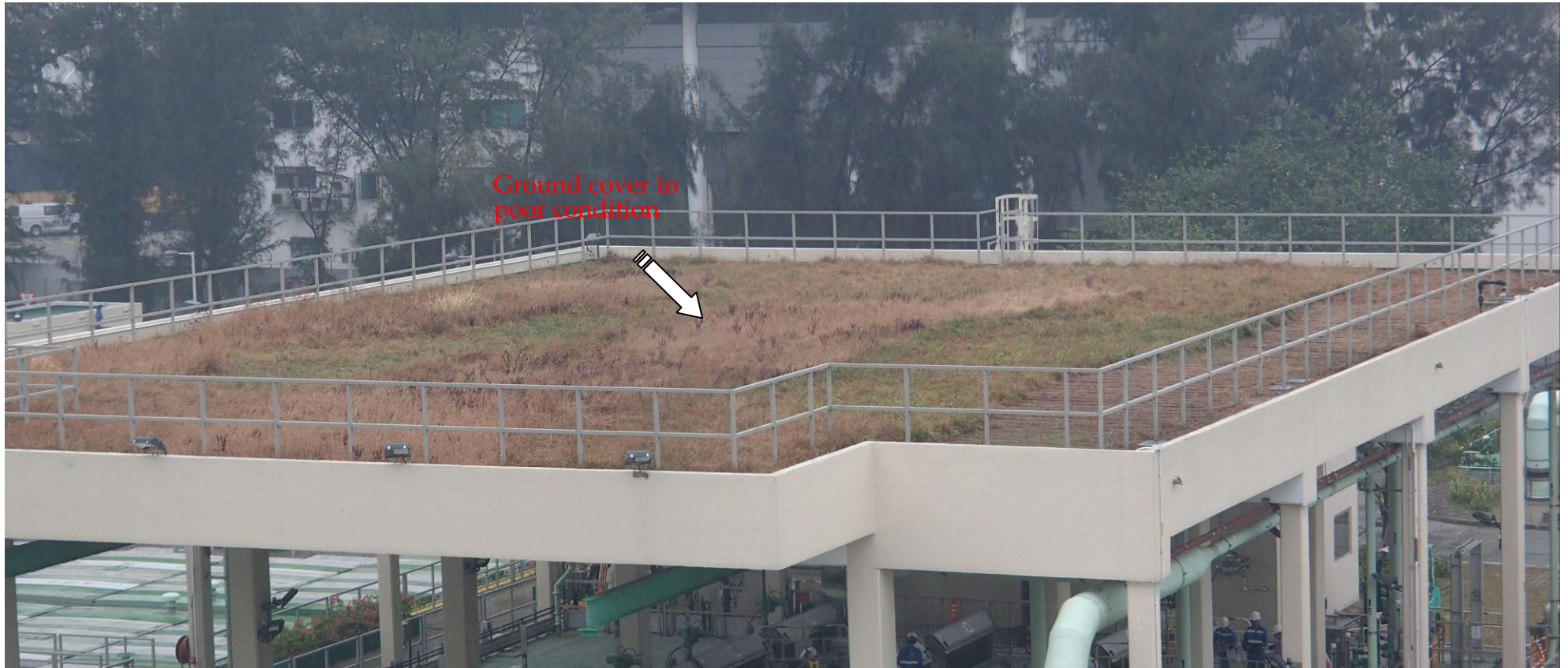
Photo no. F-02 : Groundcover & Lawn in roof garden ( CEPT Tanks ) were observed in poor condition.
