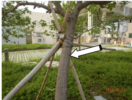
Tree tag was found damaged.
