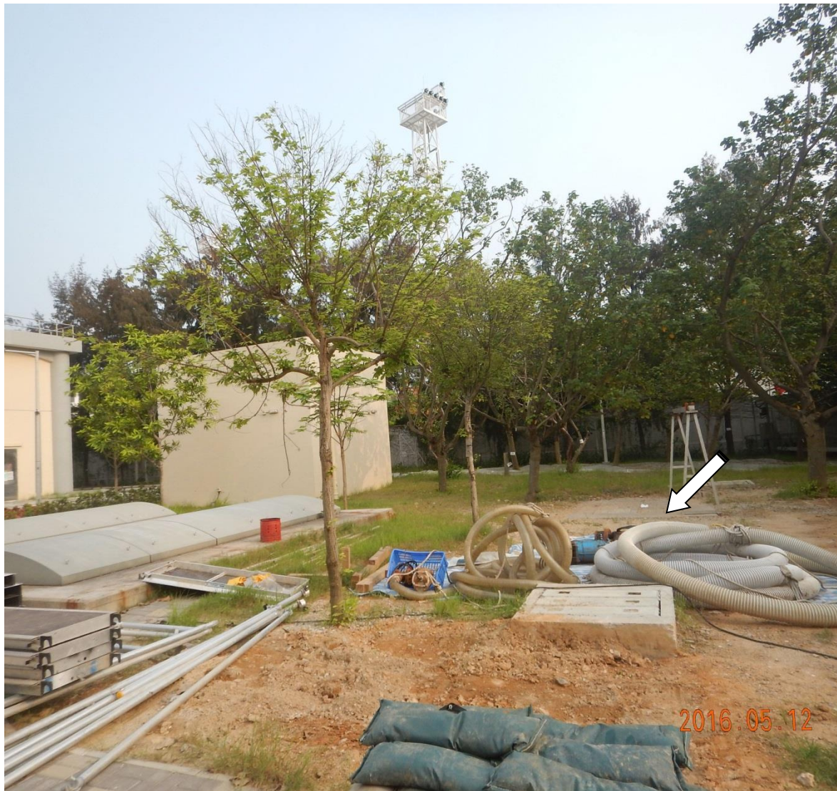
Photo no. G-10 : Groundcover and Lawn were observed missing during the site inspection.
