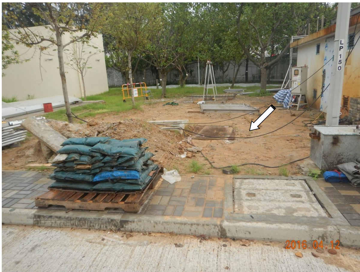
Photo no. G-13 : Groundcover and Lawn were observed missing during the site inspection.
