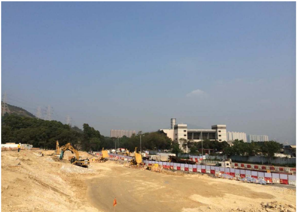
Landfill Gas Monitoring Location – Retaining Wall B
