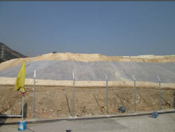
Photo 7 Covered part of the exposed slopes by geotextile net was observed on 12 December 2014.
