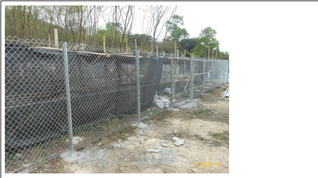
Item 1. Existing trees on boundary of the Project Area have been protected carefully during construction.
