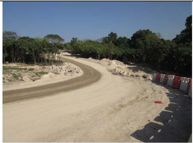
Photo 9 Water spraying was applied on haul road, however, the Contractor should increase the coverage of watering.
