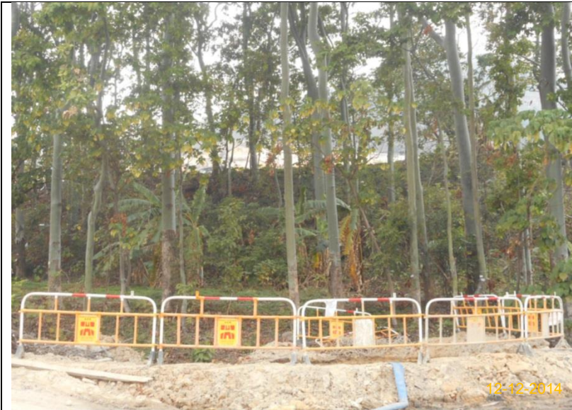
Item 1. Existing trees on boundary of the Project Area have been protected carefully during construction.
