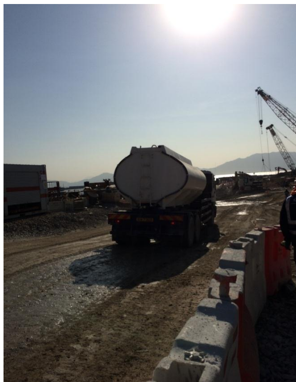
Use of water truck on exposed soil within the Project site and associated work areas. (Reclamation Works Area)
