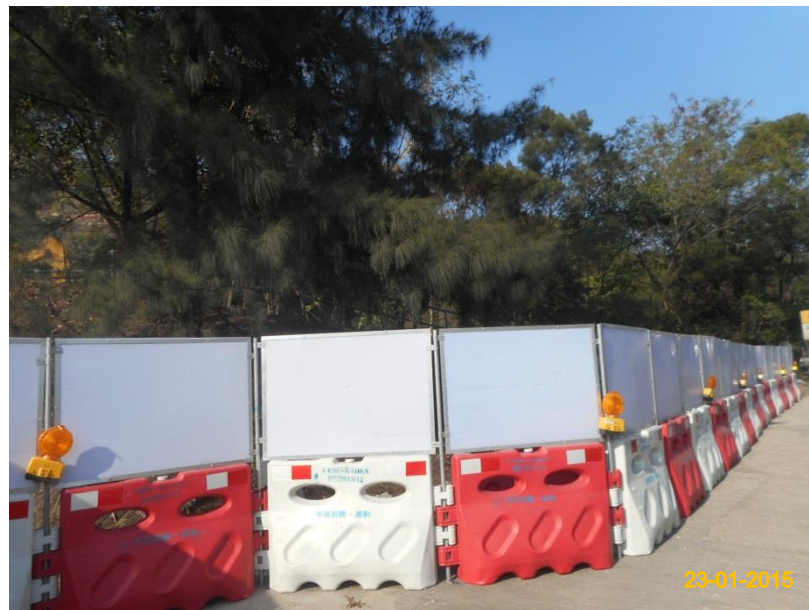
Item 5. Water Barrier with panel around works area. Item 6. Temporary traffic management lighting.
