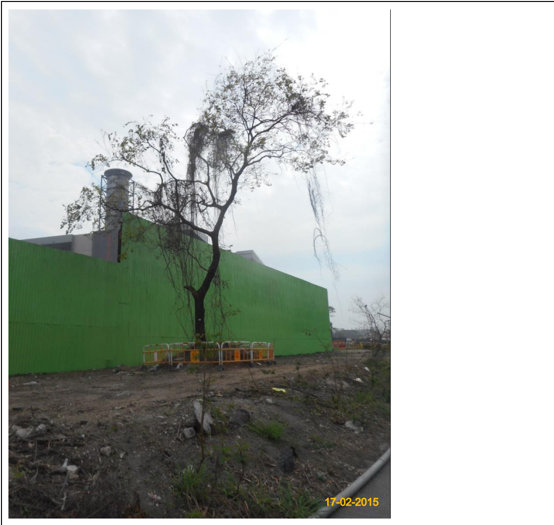
Item 1. Existing trees on boundary of the Project Area have been protected carefully during construction.
