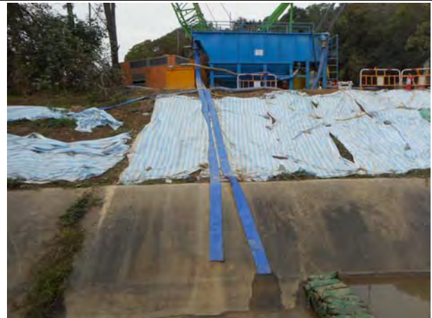
Photo 2 The wastewater from piling work was recirculated after treatment in the AquaSed and no discharge was made.
