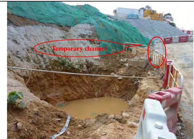
Photo 4 Sump pit with temporary channel were constructed under the slopes to divert the site runoff for temporary storage and primarily desilting before divert to the AquaSed.
