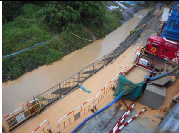
Photo 4 Run off from excavation area was flowing into the existing channel during rainstorm.
