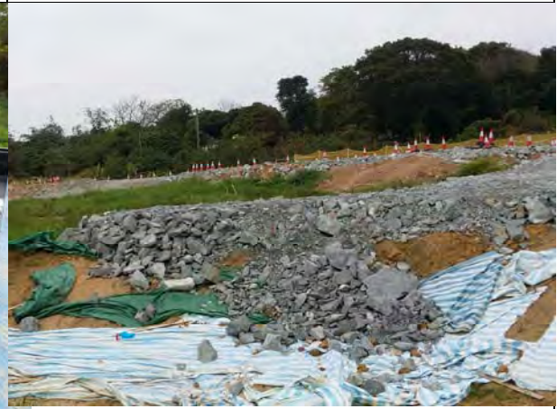
Photo 4 During site inspection in on 14 January 2016, it was observed that slope adjacent to the river course was laid with rock fill and covered with tarpaulin to minimize muddy runoff
