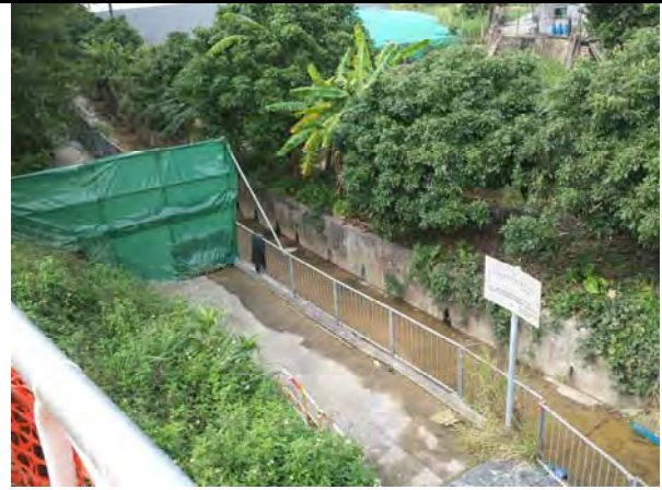
Photo 8 During site inspection on 7 January, it was observed that the channel next to the site was clear and no discharge from the site was observed
