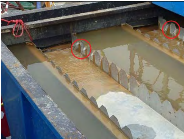
Photo 3 Self-monitoring was conducted by the Contractor and treated water in the AquaSed was acceptable. The Contractor was advised to remove the silt in the AquaSed to ensure it functions effectively.
