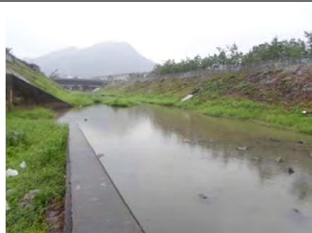
Photo 3 Turbid water was observed at WM4-CB on 15 January 2016
