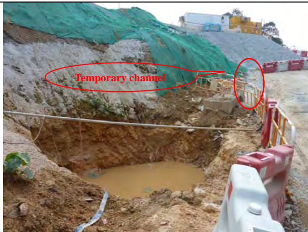
Photo 3 Sump pit with temporary channel were constructed under the slopes to divert the site runoff for temporary storage and primarily desilting before divert to the AquaSed.
