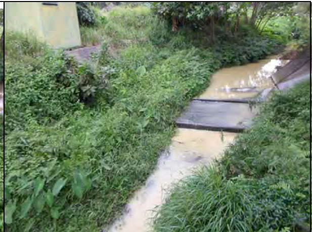
Photo 2 Turbid water was observed at WM2A during water monitoring on 18 January 2016.
