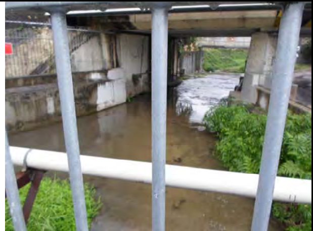
Photo 2 Turbid water was observed at WM4-CA on 15 January 2016
