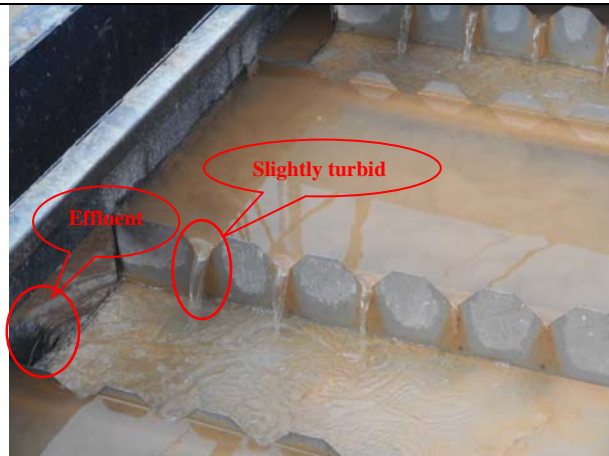
Photo 3 Self-monitoring was conducted by the Contractor on 16 January 2016 and treated water in the AquaSed was slightly turbid. As advised by the Contractor, desludging of the AquaSed is now carried out daily to ensure it functions effectively.
