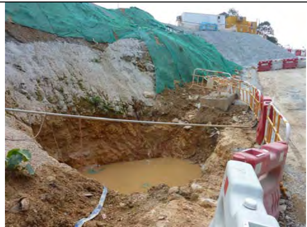
Photo 4 Sump pit with temporary channel were constructed under the slopes to divert the site runoff for temporary storage and primarily desilting before divert to the AquaSed.
