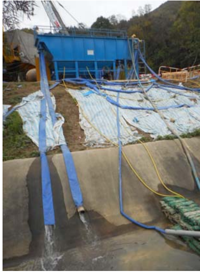
Photo 7 The effluent of the AquaSed was visually clear.
