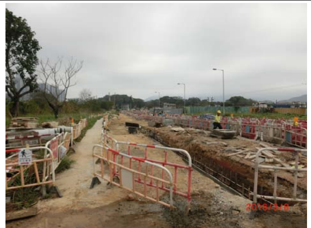
Photo 8 During site inspection on 8 March 2016, construction of u-channel was observed. No adverse water quality impact was noted.
