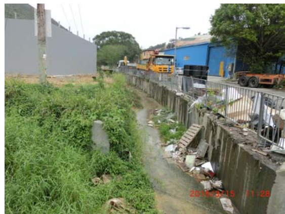
Photo 3 During water sampling on 15 March 2016, shallow water was observed at WM2B and the water quality at WM2B was visually clear.
