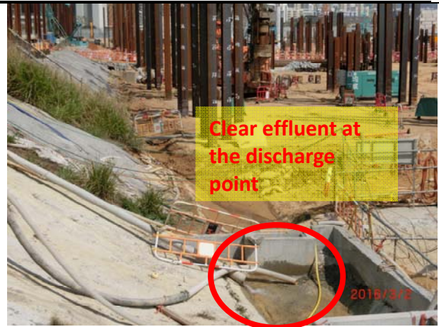
Photo 8 During site inspection on 2 March 2016, it was observed that the effluent from the AquaSed was visually clear.
