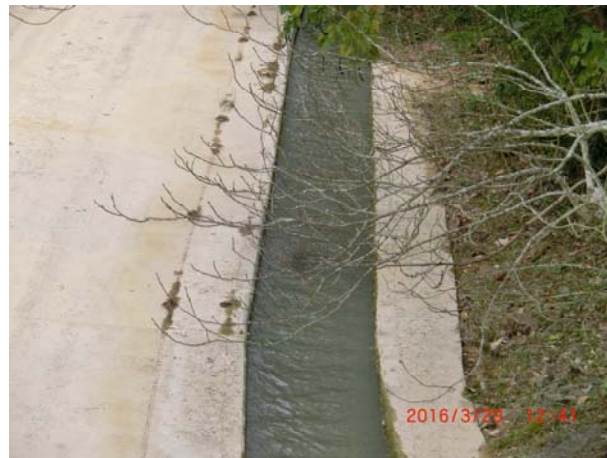
Photo 1 Muddy water was observed at WM3 on 29 March 2016
