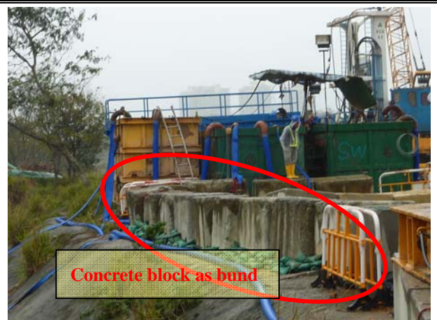
Photo 4 Wastewater treatment facilities was installed for piling work at Bridge D. Moreover, concrete block and sand bag act as a bund was provided at the area of the piling works besides of Ping Yuen River of Bridge D.
