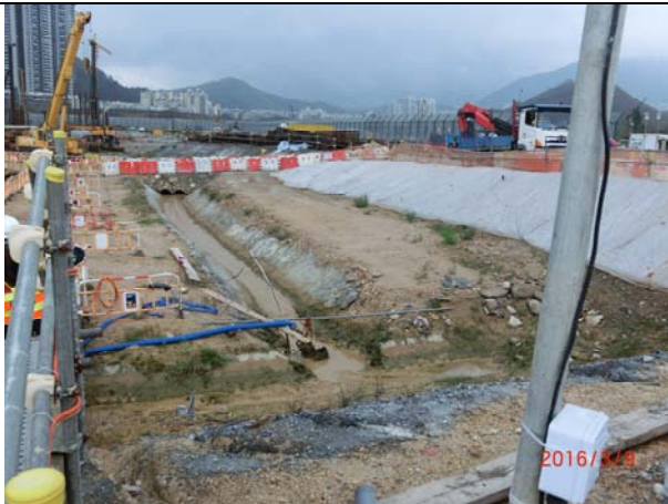
Photo 3 During site inspection on 9 March 2016, the perimeter channel was in proper function.
