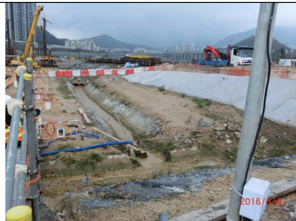
Photo 9 During site inspection on 9 March 2016, the perimeter channel was in proper function.
