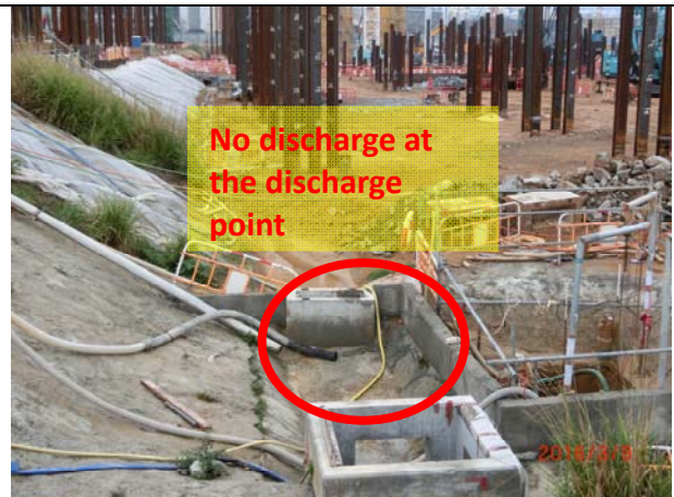
Photo 10 During site inspection on 9 March 2016, there was no discharge observed from the wastewater treatment system.
