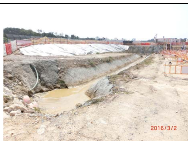
Photo 11 Temporary drainage channel has been constructing at the periphery of the site and the formation level of the site is lower than the roads bounding the site
