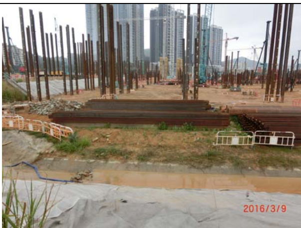
Photo 5 Temporary drainage channel has been constructing at the periphery of the site and the formation level of the site is lower than the roads bounding the site
