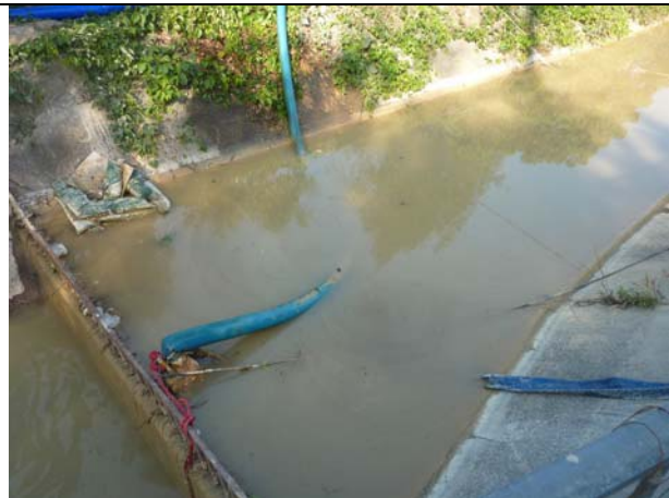
Photo 4 The muddy water in the open channel was pumped back to the AquaSed for treatment and recirculated for bored piling.
