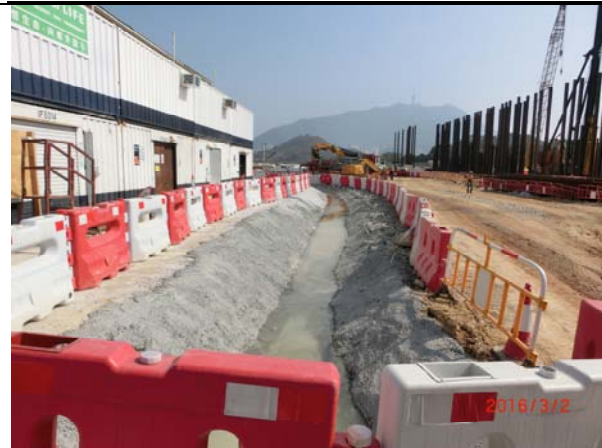
Photo 7 During site inspection on 2 March 2016, the perimeter channel was in proper function.
