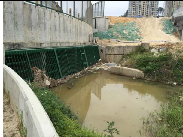
Photo 1 During water sampling on 4 March 2016, turbid water was observed at WM1.
