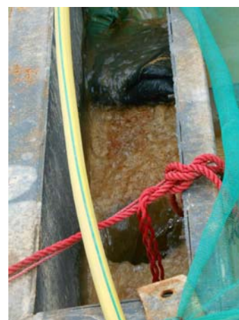
Photo 6 The effluent of the AquaSed was visually clear.
