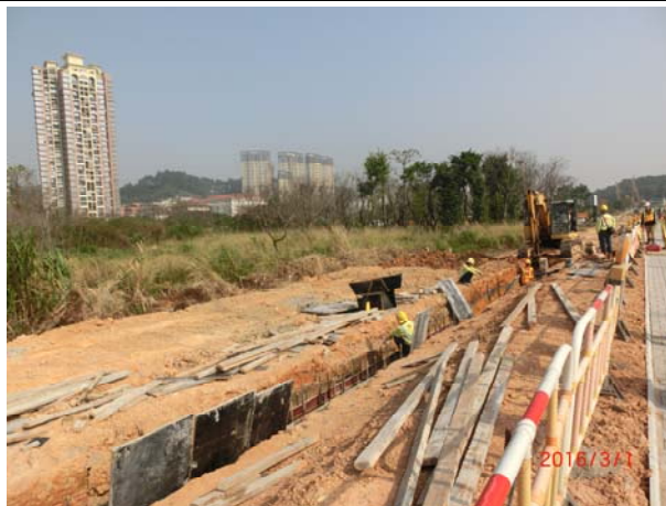
Photo 7 During site inspection on 1 March 2016, construction of u-channel was observed. No adverse water quality impact was noted.
