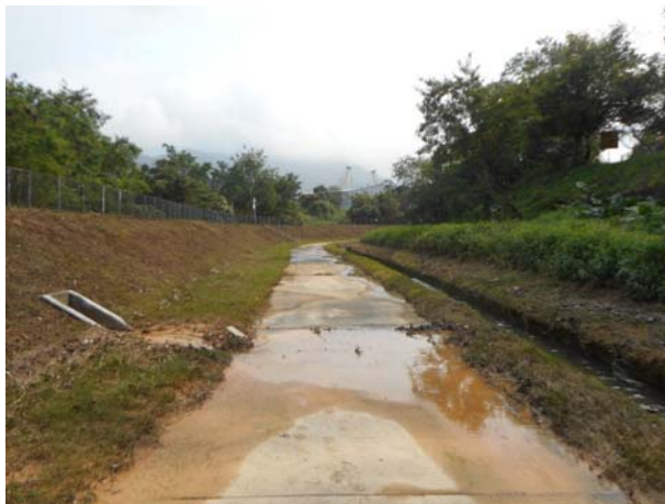
Photo 7 Discharge of turbid water and accumulated silt was observed from an unknown outfall which located at between the works area of C6 and WM3 on 29 March 2016.
