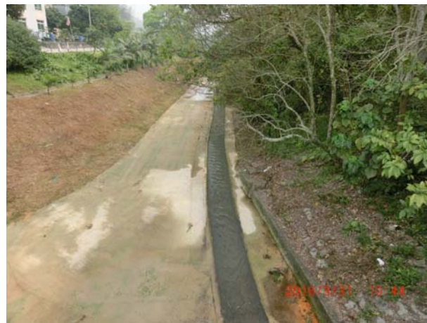
Photo 3 Muddy water was observed at WM3 on 31 March 2016
