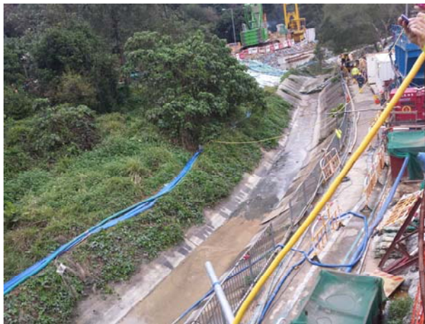
Photo 9 During site inspection on 10 March 2016, it was observed desilting work at upstream portion was completed
