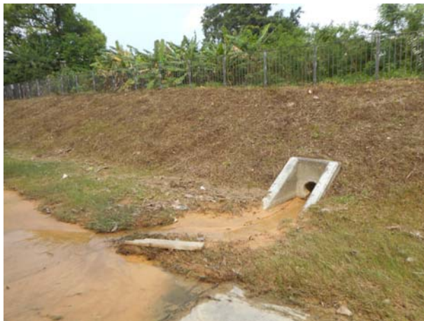
Photo 9 Discharge of turbid water and accumulated silt was observed from an unknown outfall which located at between the works area of C6 and WM3 on 31 March 2016.
