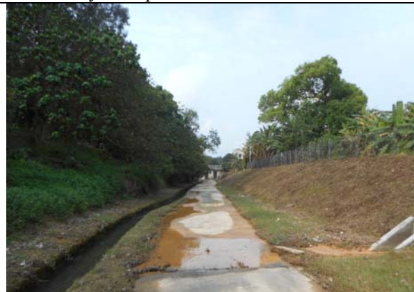
Photo 5 Discharge of turbid water and accumulated silt was observed from an unknown outfall which located at between the works area of C6 and WM3 on 2 April 2016.
