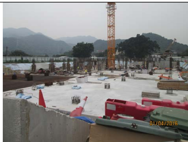
Photo 3 During weekly site inspection on 1 April 2016, it was observed that building foundation works was carried out at Admin Building and the site area was mostly hard paved.
