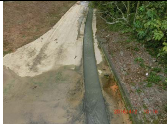
Photo 1 Turbid water was observed at WM3 on 2 April 2016.
