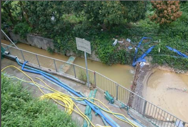
Photo 3 The silt cumulated at the channel bed was blocked by the bar screen to prevent it getting to downstream. However, it was disturbed by the flow of discharge from the AquaSed and the mixture of silt and discharge water was overflow to the downstream.
