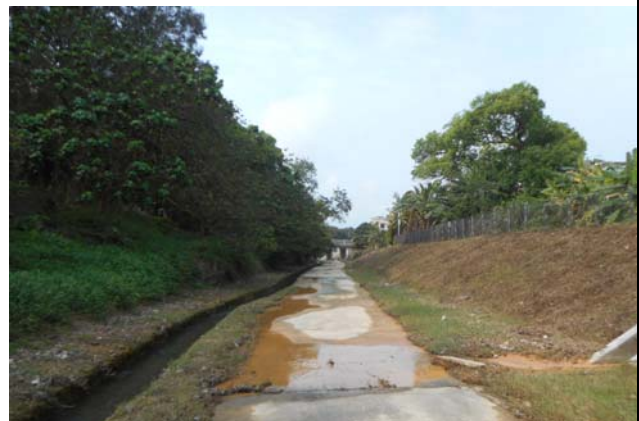
Photo 4 Discharge of turbid water and accumulated silt was observed from an unknown outfall which located between the works area of C6 and WM3 on 2 April 2016.
