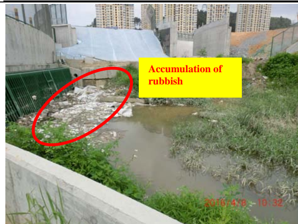
Photo 13 During water sampling on 8 April 2016, accumulation of rubbish were observed at the bar screen of the box culvert near WM1 and cumulated turbid water was observed at WM1.
