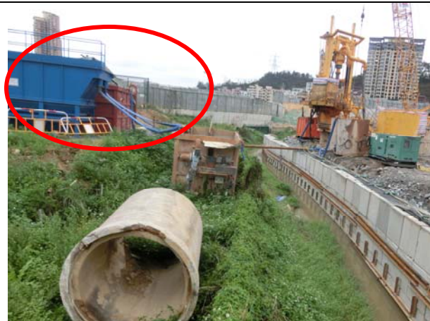
Photo 17 During site inspection by the RE, IEC, Contractor and ET on 7 April 2016, it was observed that the wastewater treatment facility was properly in place and function.
