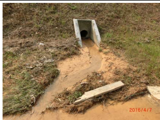
Photo 6 Accumulated silt was observed from an unknown outfall which located at between the works area of C6 and WM3 on 7 April 2016.
