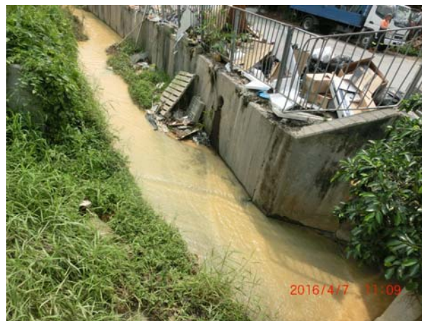
Photo 1 During water sampling on 7 April 2016, it was observed that the water at WM2B was turbid.
