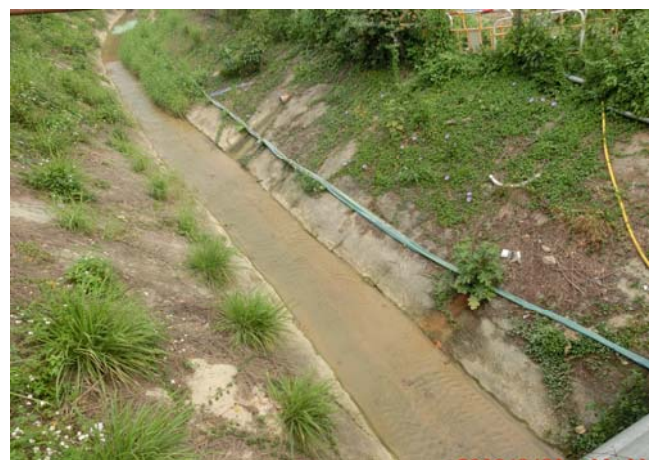
Photo 6 Though some silt cumulated at nullah bed was observed on 31 March 2016, the water flowing in the nullah was visually clear.
