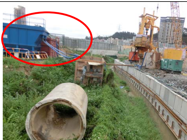
Photo 5 During site inspection by the RE, IEC, Contractor and ET on 14 April 2016, it was observed that the wastewater treatment facility was properly in place and function.
