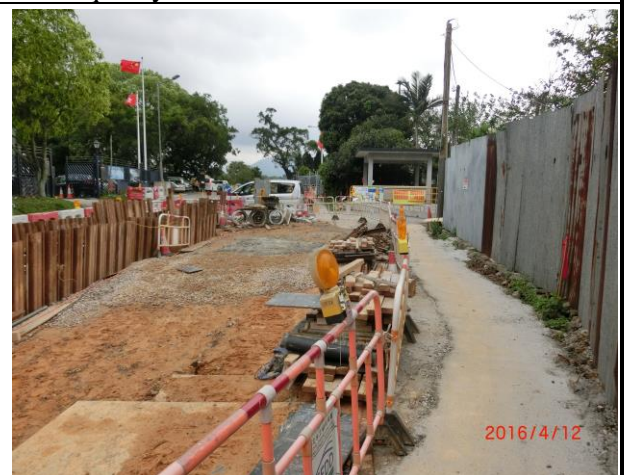
Photo 4 During site inspection on 12 April 2016, construction of u-channel and bituminous laying were observed. No adverse water quality impact was noted.
