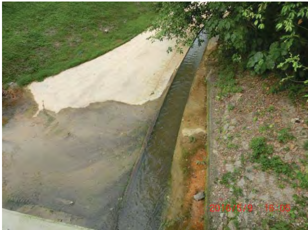
Photo 1 Visually clear water was observed at WM3 on 9 May 2016.
