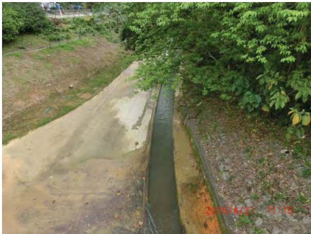
Photo 3 Slightly turbid water was observed at WM3 on 21 April 2016.
