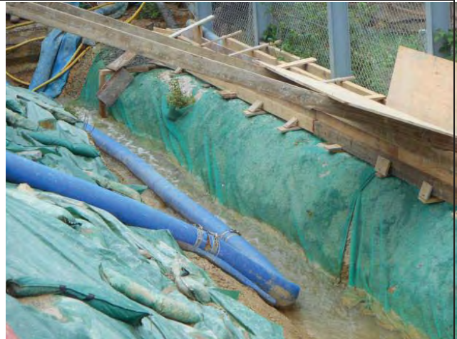
Photo 8 After the replenishment of the flocculent, the effluent observed was clear.
