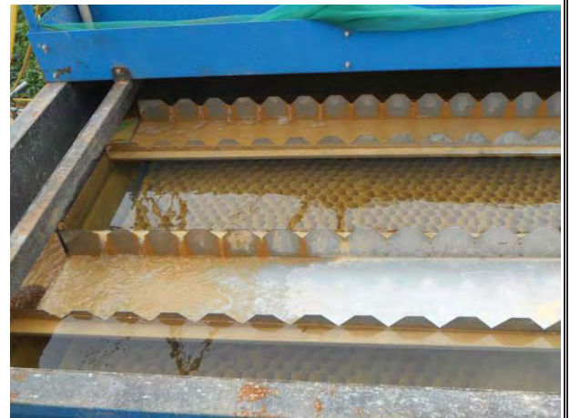
Photo 4 The effluent of the AquaSed on 20 April 2016 was visually clear.
