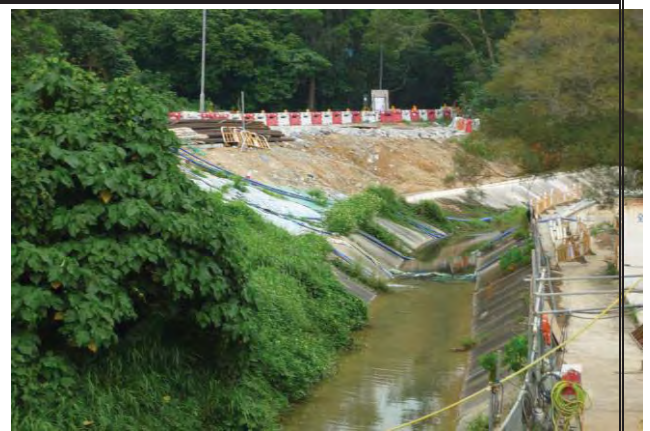
Photo 6 During joint site inspection on 12 May 2016, no adverse water impact was observed at upper stream of WM2B.
