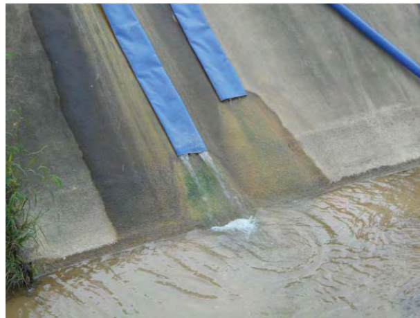
Photo 3 The effluent of the AquaSed on 20 April 2016 was visually clear.
