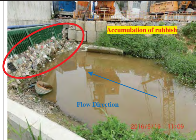
Photo 4 During water sampling on 19 May 2016, accumulation of rubbish were observed at the Box Culvert in WM1.
