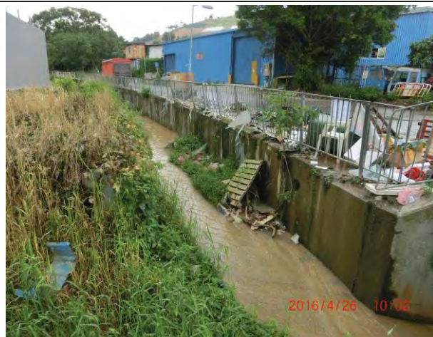
Photo 7 During water sampling on 26 April 2016, it was observed that the water at WM2B was turbid.
