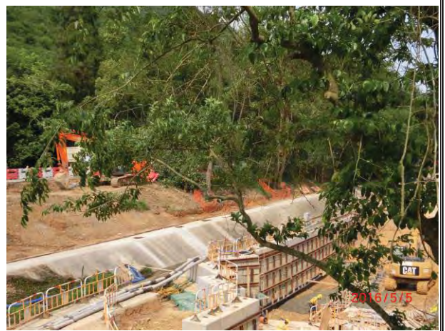
Photo 12 During site investigation on 5 May 2016, no runoff was observed after the completion of the temporary drain ditch.
