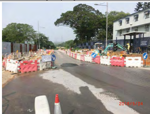
Photo 9 Bituminous laying works was undertaking. No adverse water quality impact was noted.
