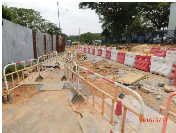
Photo 7 Bituminous laying works was undertaking. No adverse water quality impact was noted.
