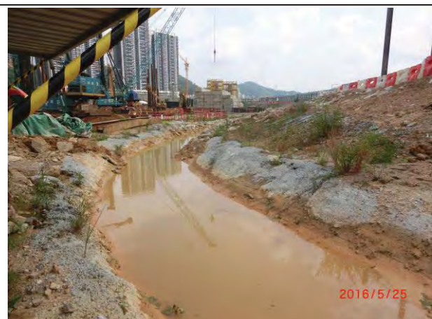
Photo 6 Temporary drainage channel has been constructing at the periphery of the site and the formation level of the site is lower than the roads bounding the site.
