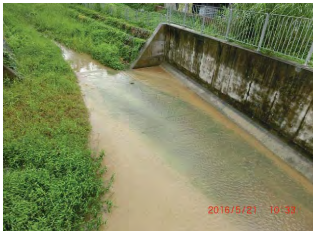
Photo 3 Slightly turbid water was observed at WM3-C on 21 May 2016.
