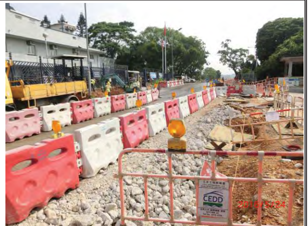
Photo 8 Bituminous laying works was undertaking. No adverse water quality impact was noted.
