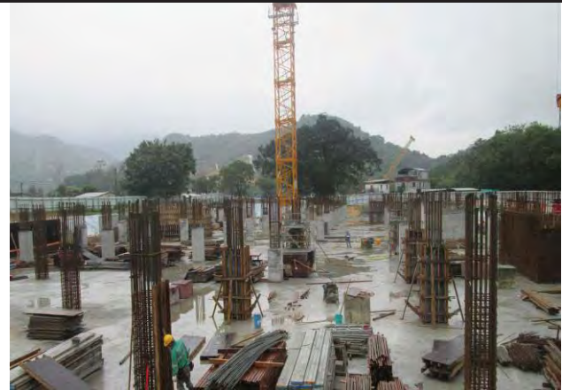
Photo 4 Building foundation works was carried out at Admin Building and the site area was mostly hard paved.
