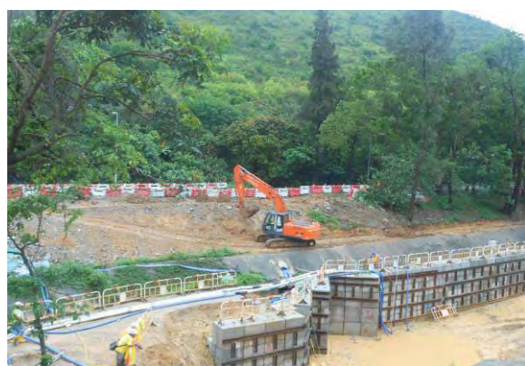
Photo 9 Runoff due to the heavy rain was generated from the loose surface where the temporary drain ditch has not been fully constructed yet, into the river channel.
