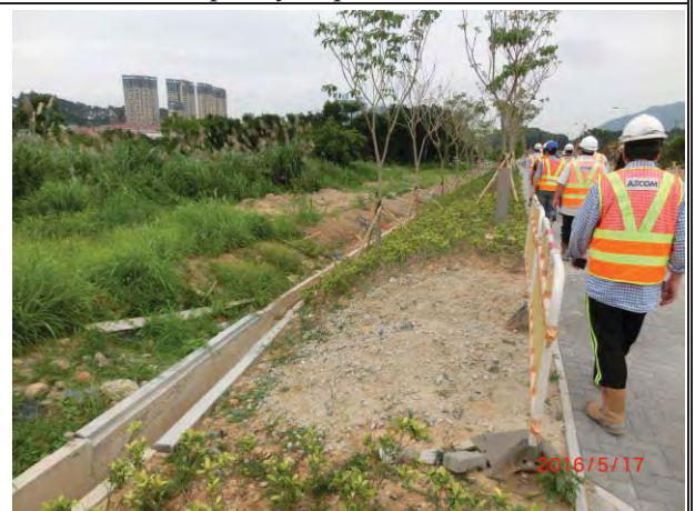
Photo 10 Construction of u-channel was observed. No adverse water quality impact was noted.
