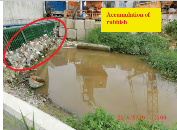
Photo 4 During water sampling on 19 May 2016, accumulation of rubbish was observed at the Box Culvert at WM1.
