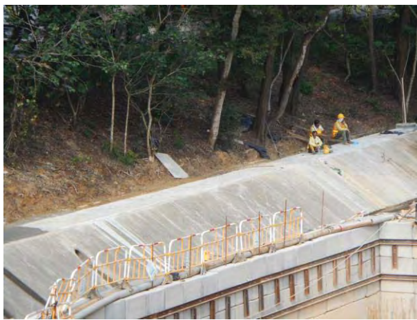
Photo 11 No runoff was observed after the completion of the temporary drain ditch.
