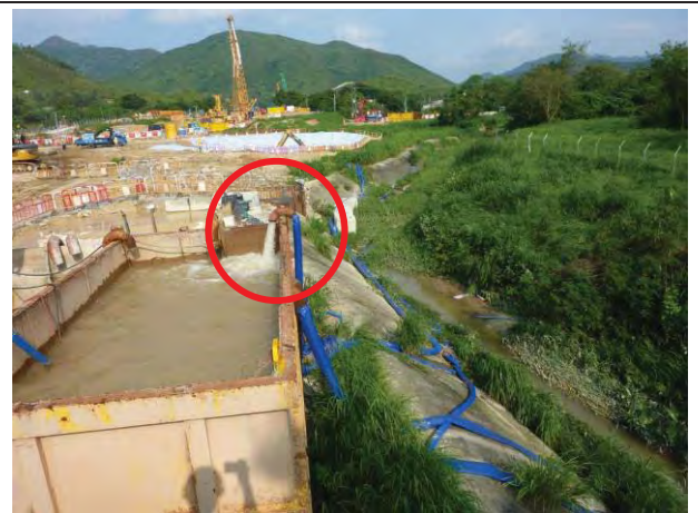
Photo 4 The inlet pipe which carried wastewater collected from the sites was incorrectly connected to the tank which received effluent from the AquaSed(SH-15).
