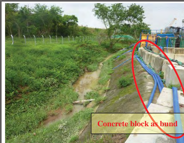
Photo 3 During weekly site inspection on 26 May 2016, it was observed that concrete block and sand bag as temporary bund was set up near the piling works which besides Ping Yuen River of Bridge D to control runoff.
