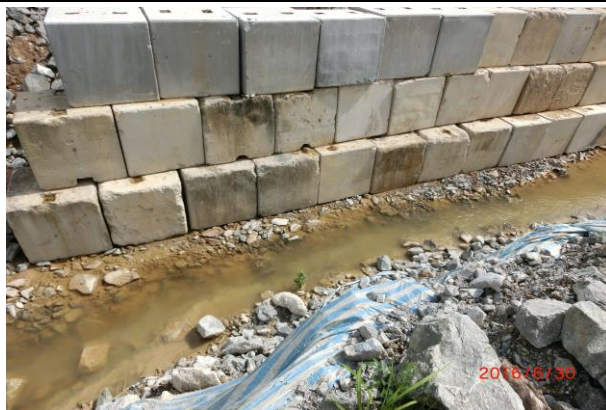
Photo 5 During joint site inspection on 30 June 2016, it was observed that unknown source of turbid water was seeping out from the river bed.
