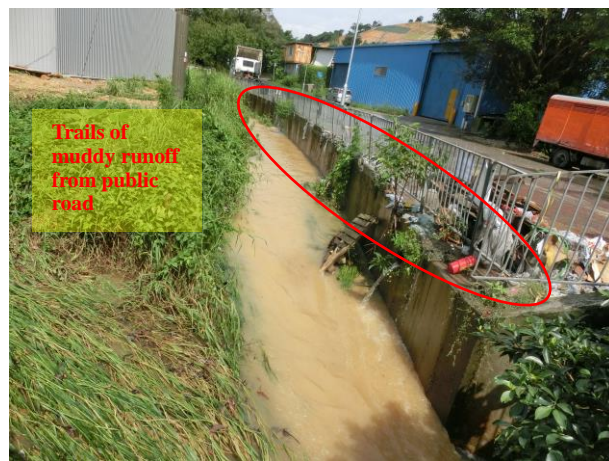
Photo 1 During water sampling on 6 June 2016, it was observed that water at WM2B was turbid. Trails of muddy road surface runoff was observed.
