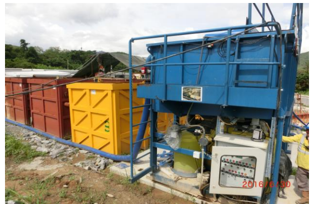
Photo 4 Wastewater treatment facilities including one AquaSed and three series of sedimentation tank have been installed for piling work.
