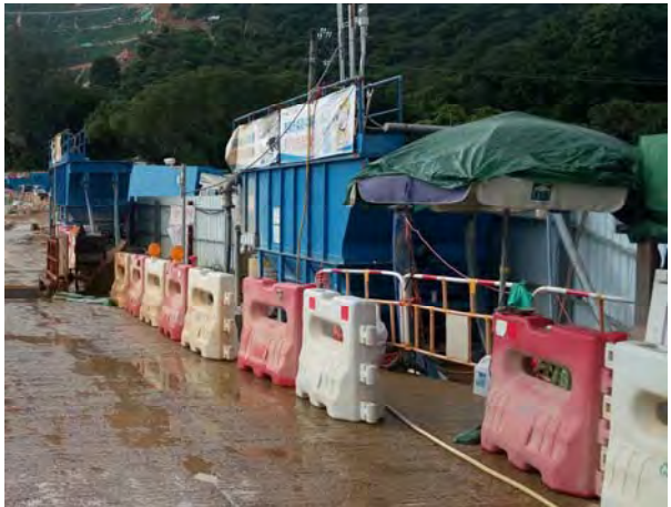
Photo 3 Wastewater treatment facilities was provided for South Portal
