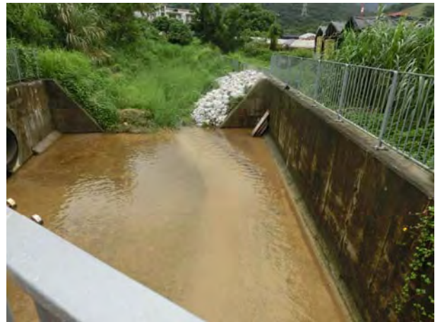
Photo 2 Turbid water was observed at WM3-C on 8 September 2016.
