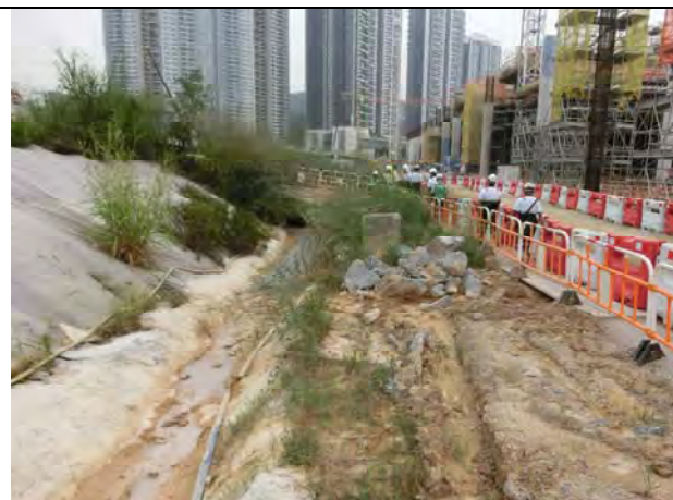
Photo 6 Temporary drainage channel has been constructing at the periphery of the site and the formation level of the site is lower than the roads bounding the site.
