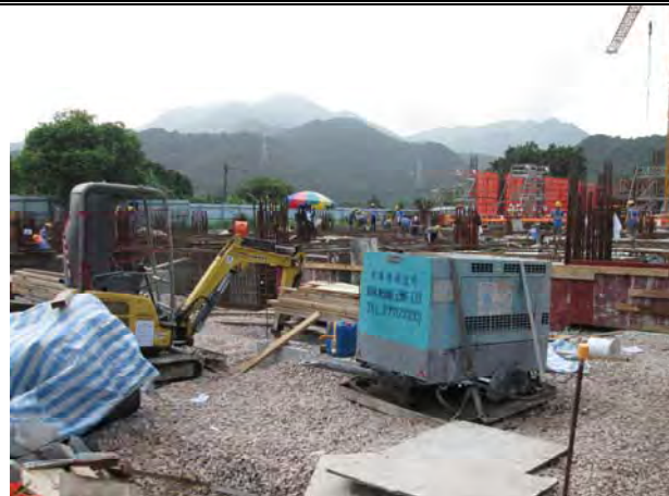
Photo 3 Superstructure works for Admin Building was carried out at Admin Building and the site area was mostly hard paved and no adverse water impact was observed.
