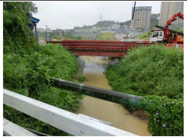
Photo 4 On 10 September 2016, muddy water was observed throughout the channel. (far outside site boundary)
