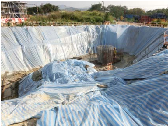
Photo 3 Works at Bridge D was mainly bridge column and pier construction and there was no discharge due to nature of works.
