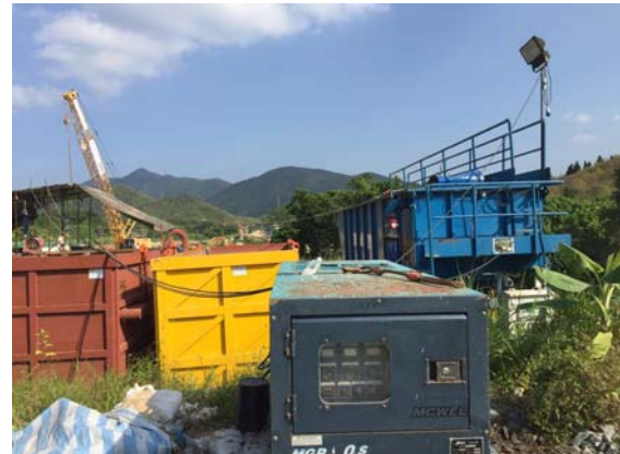
Photo 4 Wastewater treatment facilities were provided for Bridge D
