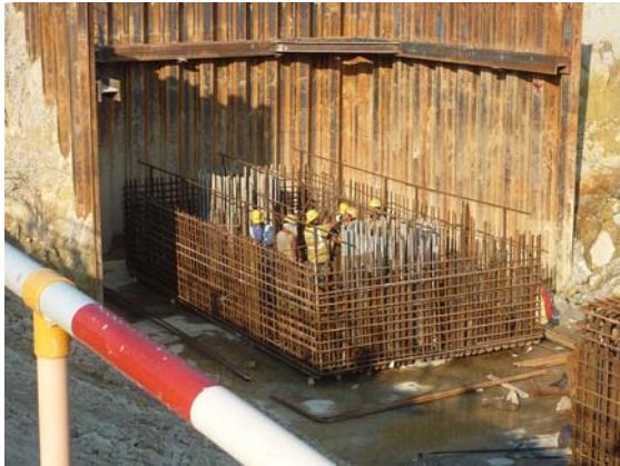
Photo 7 Works at Bridge D was mainly bridge column and pier construction and there was no discharge due to nature of works.
