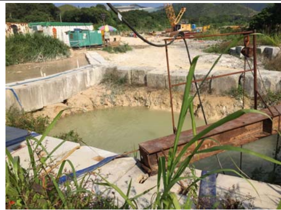
Photo 10 A sump pit was constructed to preliminary settled the particulates in the water before diverted to the AquaSed for proper treatment.
