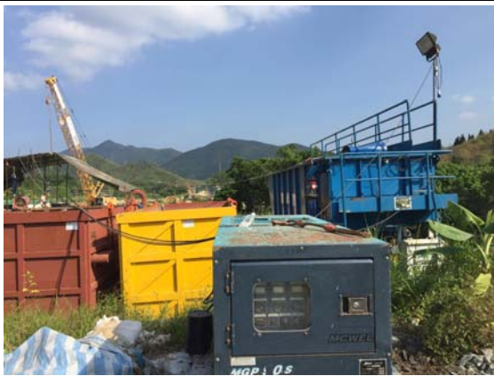
Photo 9 Wastewater treatment facilities were provided for Bridge D
