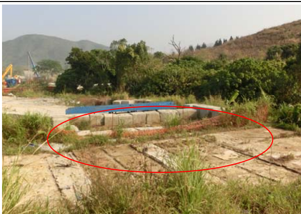
Photo 11 To minimize the muddy runoff from the site, concrete block as temporary bund was provided align the river course and no turbid runoff and discharge was made from the site.
