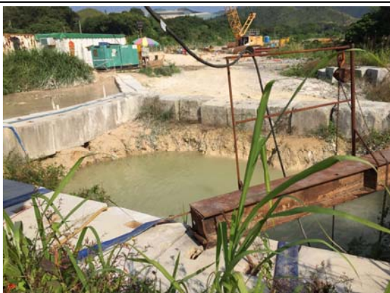
Photo 5 A sump pit was constructed to preliminary settled the particulates in the water before diverted to the AquaSed for proper treatment.
