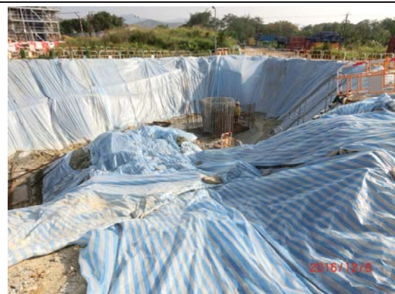
Photo 12 The Contractor has covered the exposed slopes as far as practicable to minimize muddy runoff.
