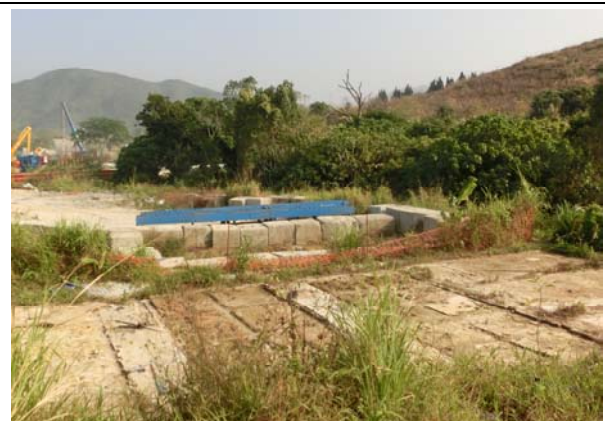
Photo 6 To minimize the muddy runoff from the site, concrete block as temporary bund was provided align the river course and no turbid runoff and discharge was made from the site.
