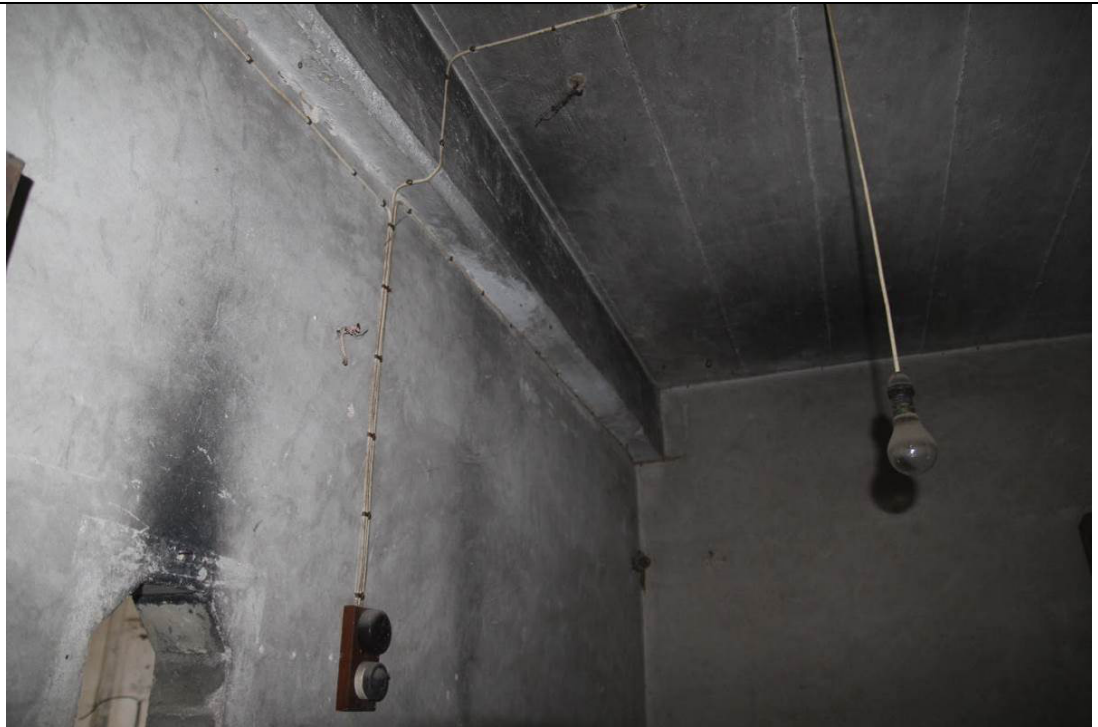
BS64-3-P34 Beam view from room under the cockloft 閣樓下房間的橫樑
