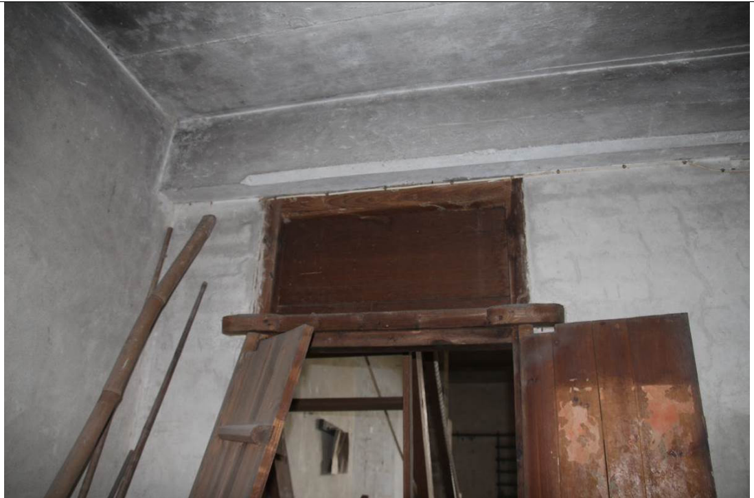
BS64-3-P35 Room door observed from room, beam has decoration 房間中看房門，橫樑上有裝飾
