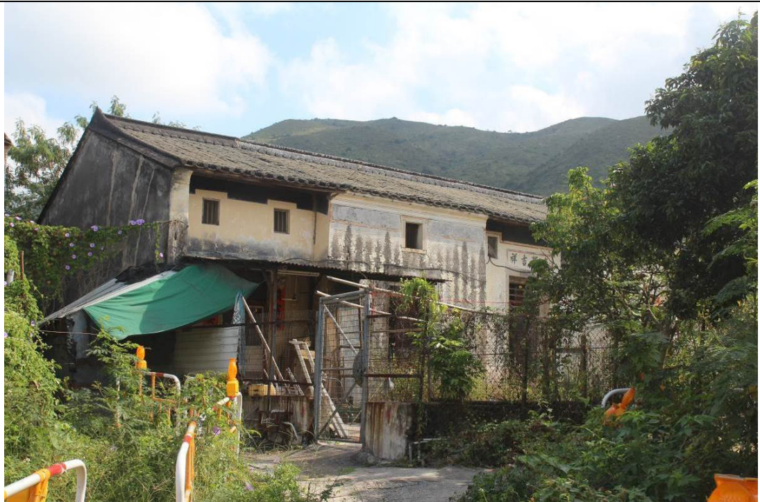
BS65-overall-P2 Oblique view of BS65 (view from northwest) BS65側視圖(攝自西北方)
