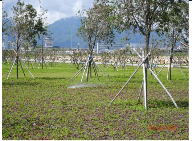
Watering system at Zone 6
