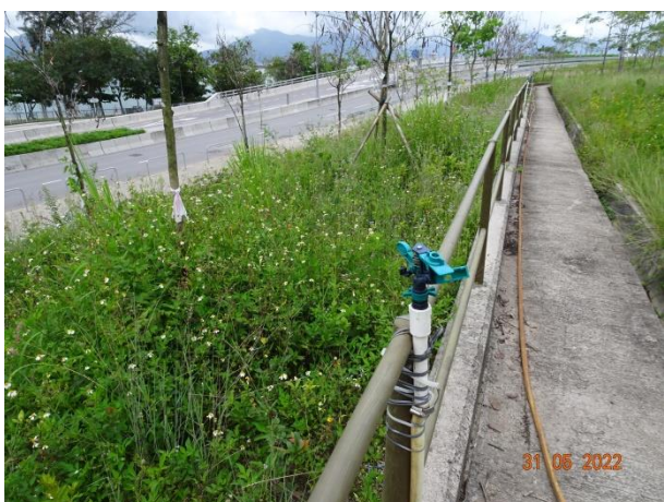
Watering system at Slope 5SE-D/C215
