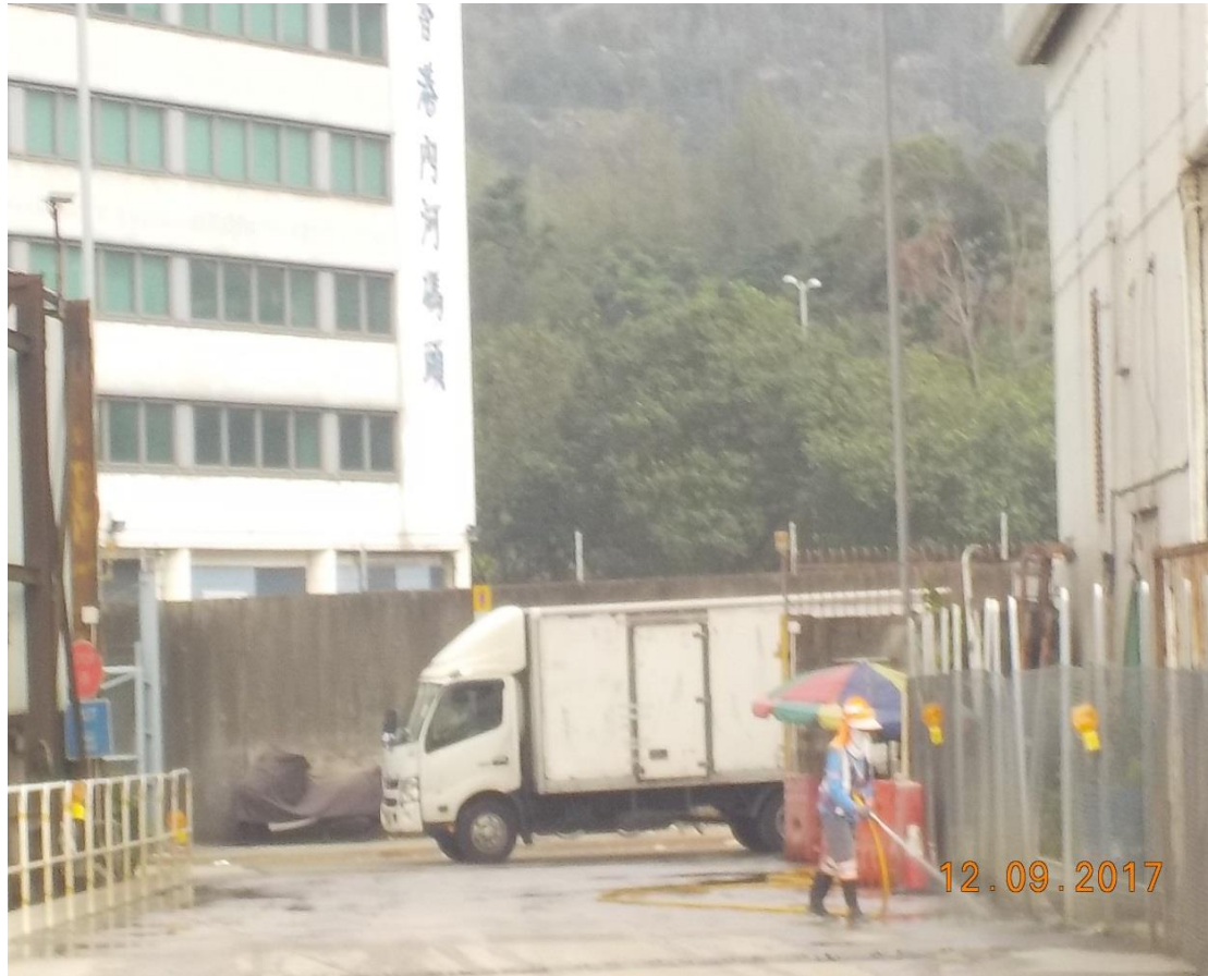
Water spraying was applied frequently during dry conditions. (Works Area Portion N-A)
