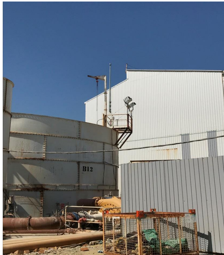
Direction of the lighting at STP is adjusted towards the ground.(After)
