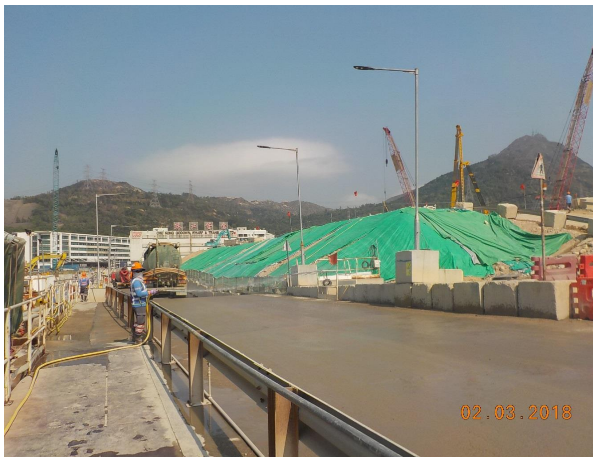
Exposed soil at Portion N-A was covered by tarpaulin sheets. (Works Area Portion N-A)
