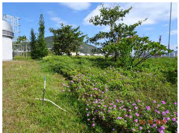
Watering System at Zone 1
