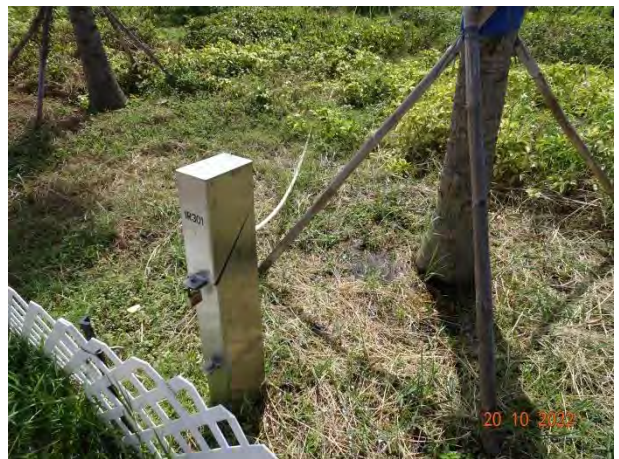
Watering system at Zone 4
