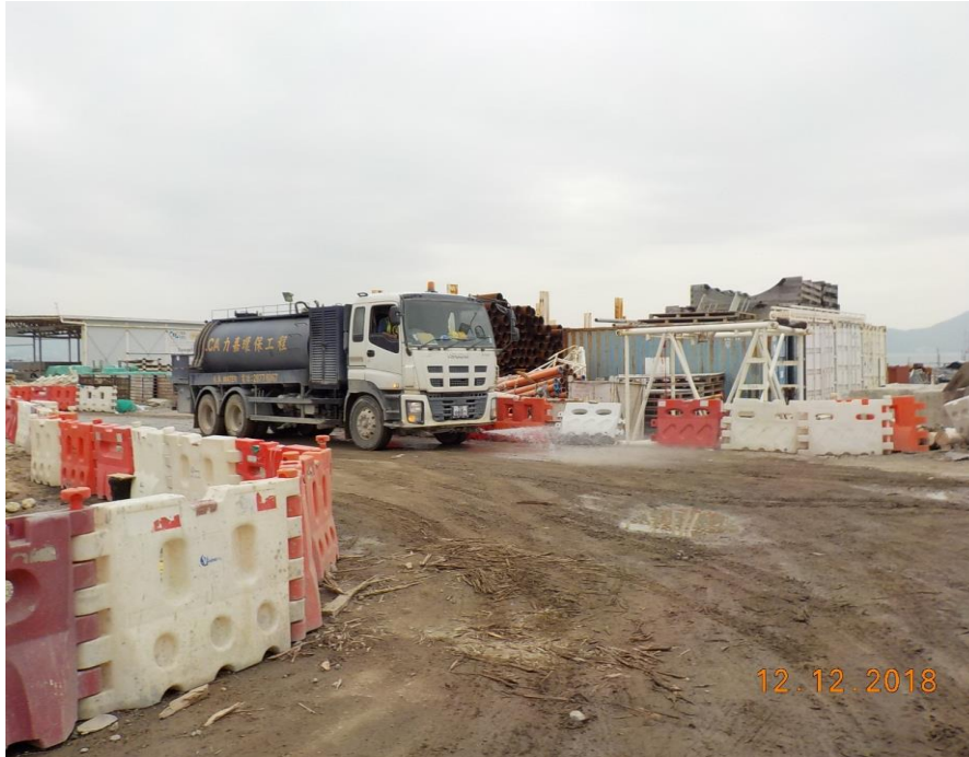
Water truck was used for dust control during surcharge removal. (Works Area Portion N-C)
