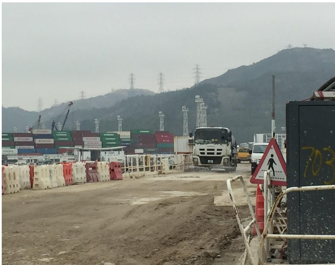
Water truck is used for water spraying at works area. (Works Area Portion N-C)
