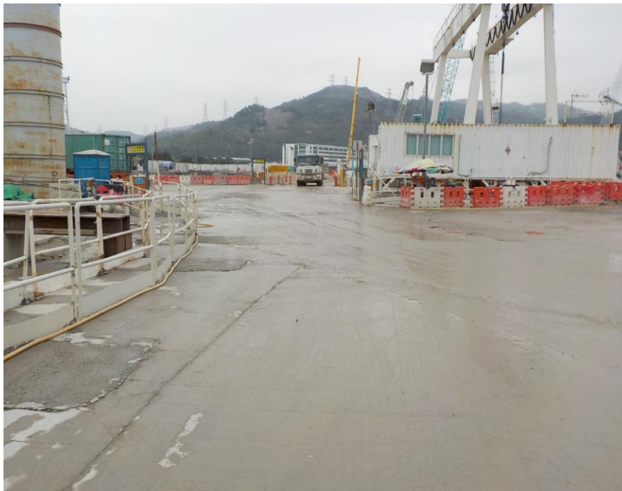
Water spraying was applied on the main haul road. (Works Area Portion N-C)
