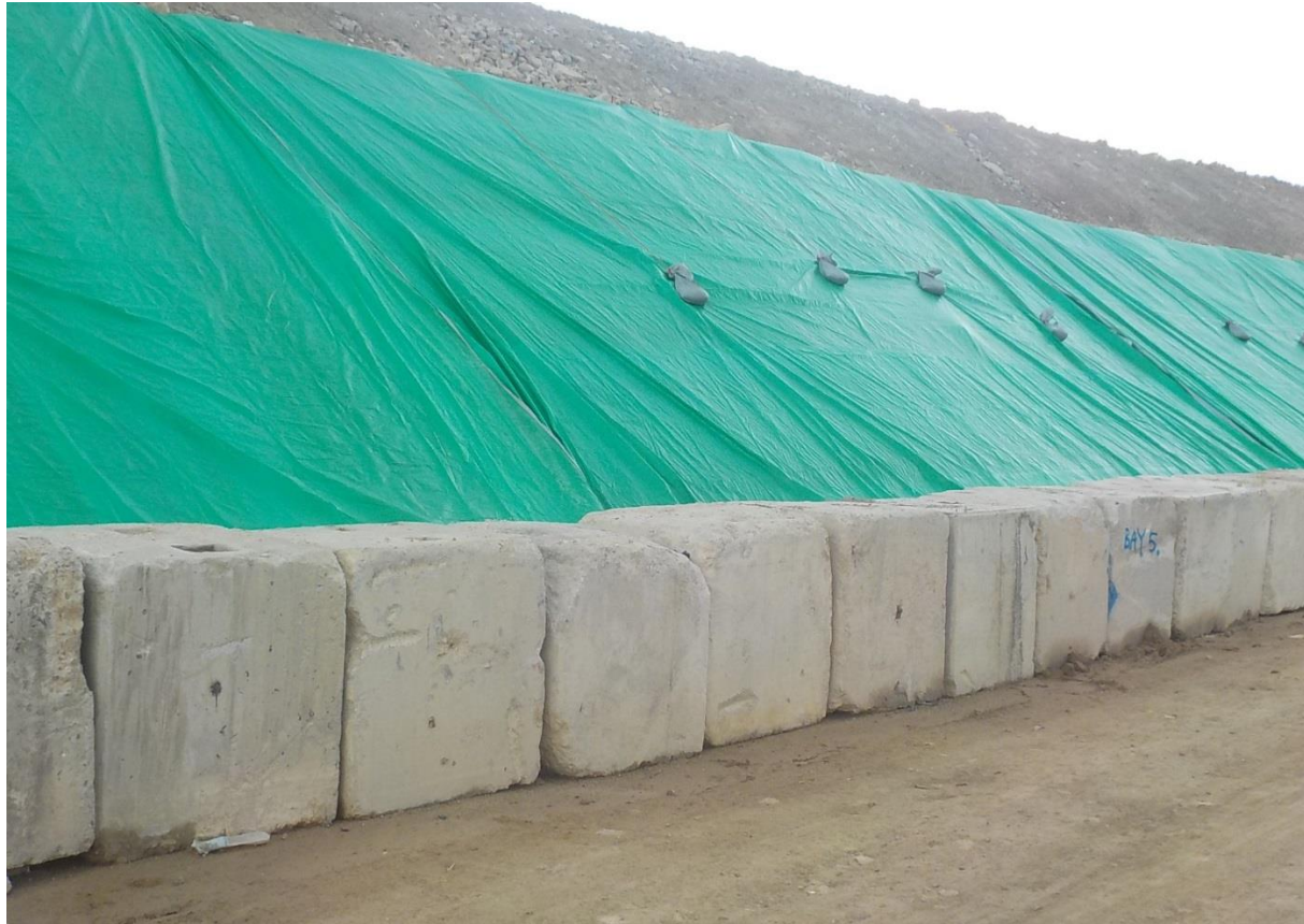
Exposed soil was covered by tarpaulin sheet to prevent dust. (Works Area Portion N-C)
