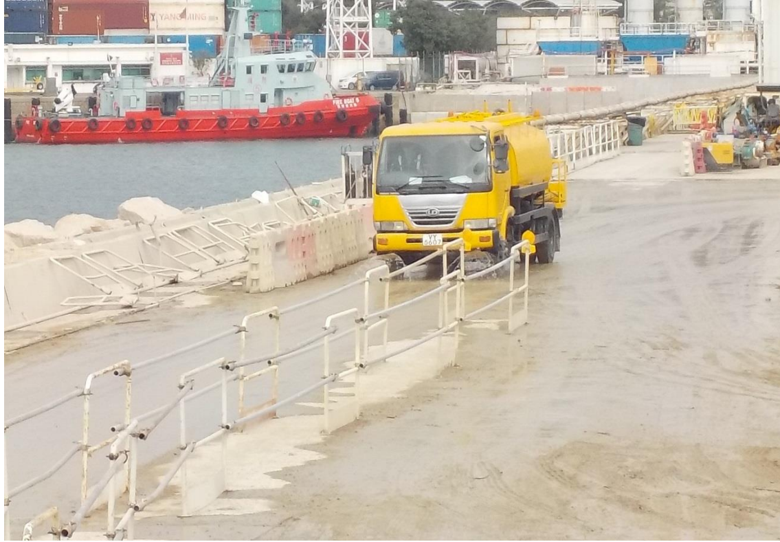
Water truck was used for water spraying to prevent dust. (Works Area Portion N-A)
