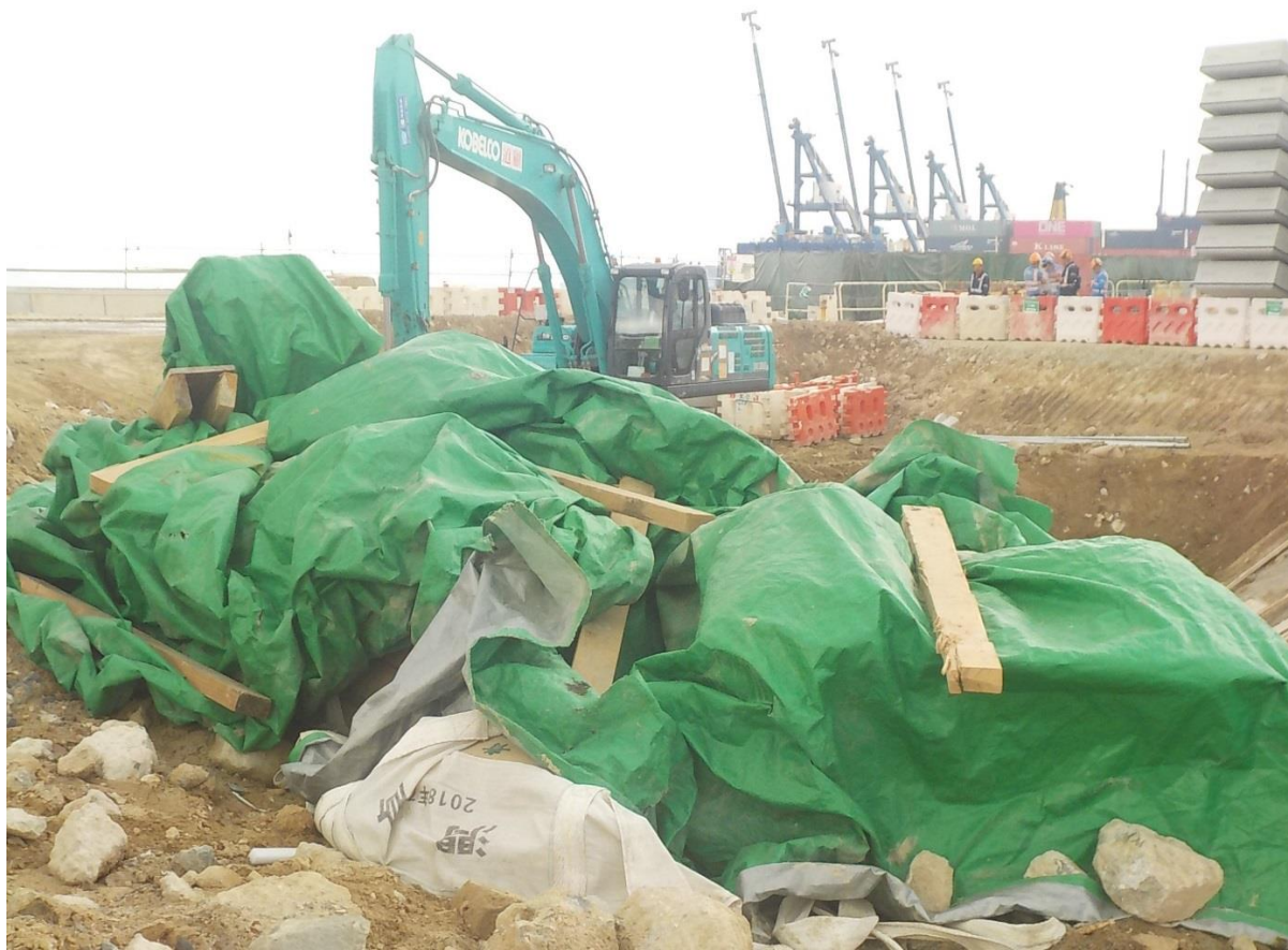
Exposed soil was covered by tarpaulin sheet to prevent dust. (Works Area Portion N-C)
