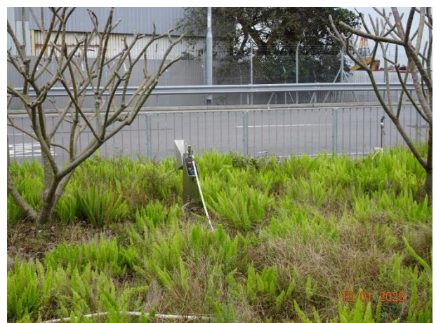
Watering System at Zone 1
