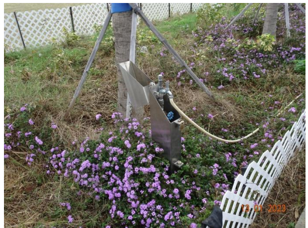
Watering system at Zone 4
