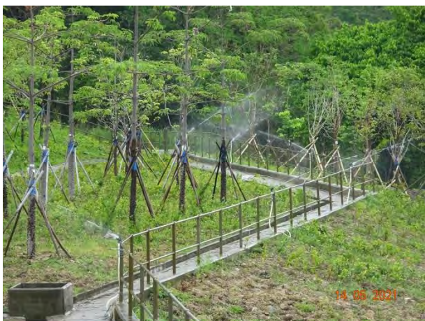
Watering system at Slope 5SE-D/C215
