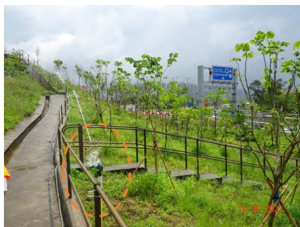
Watering system at Slope 5SE-D/C170
