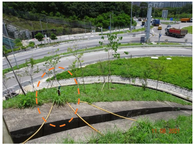
Watering system at Slope 5SE-D/C170
