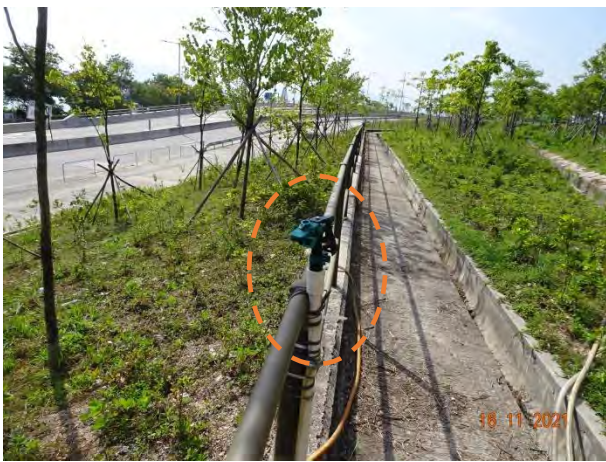
Watering system at Slope 5SE-D/C215
