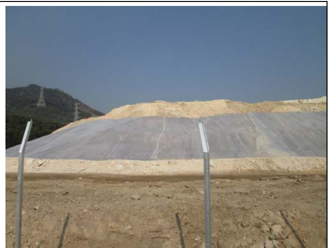
Photo 5 Covering of the exposed slopes by geotextile net was observed on 9 December 2014.
