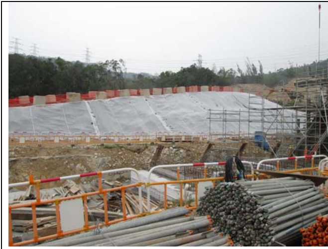
Photo 4 Covering of the exposed slopes by geotextile net was observed on 2 December 2014.
