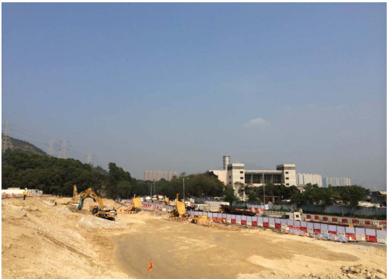
Landfill Gas Monitoring Location – Retaining Wall B
