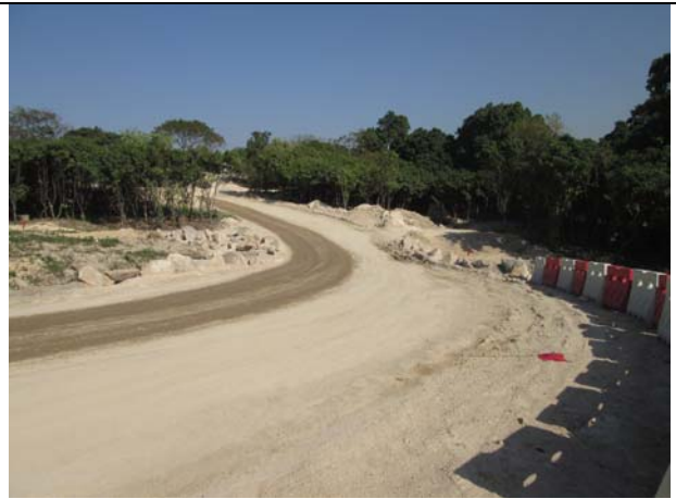
Photo 9 Water spraying was applied on haul road, however, the Contractor should increase the coverage of watering.
