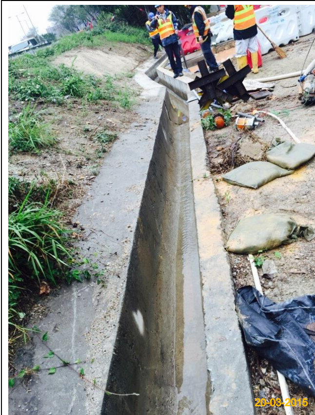
Item 7. Ensure no run-off into water body during rainy days.
