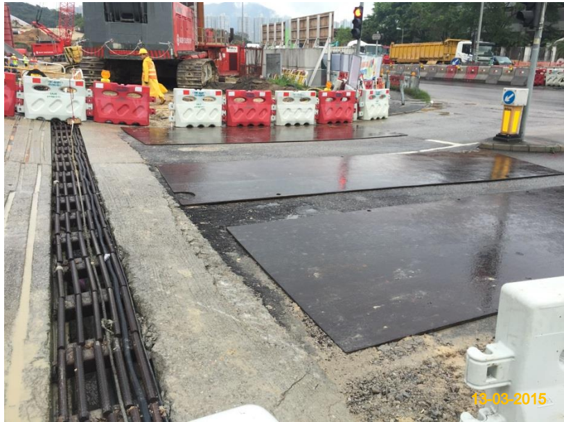
Item 7. Ensure no run-off into water body during rainy days.
