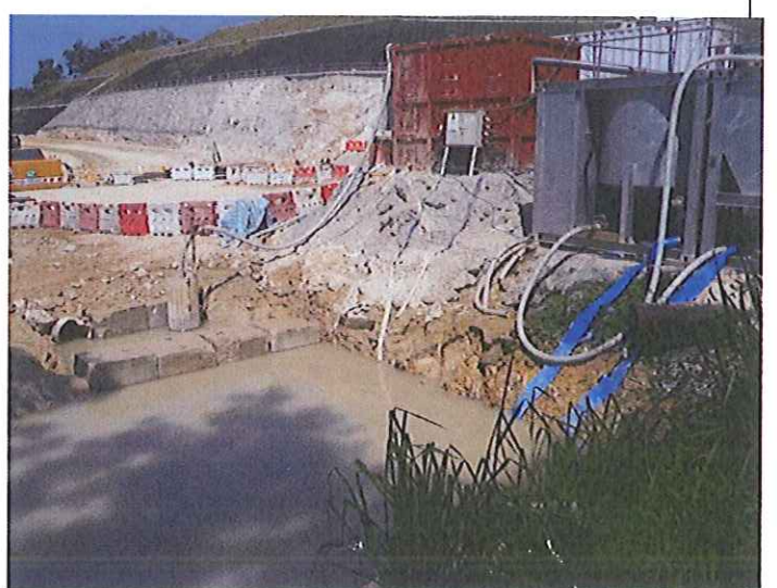
Wastewater treatment facilities were provided.
