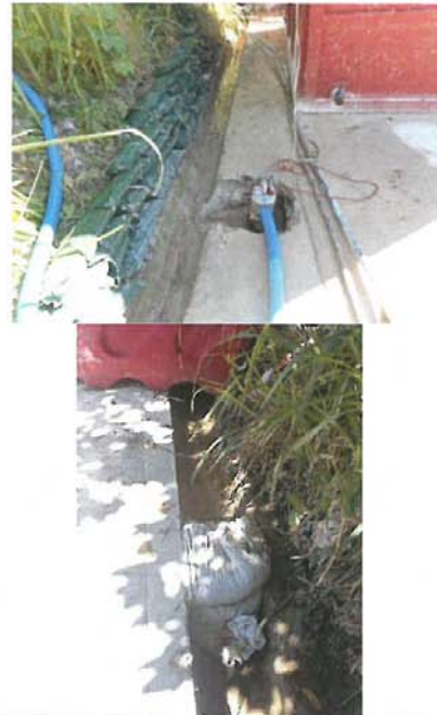
Photo 4a: The u-channel was cleaned. Sand bags were provided to protect the u-channel and sump pit was provided to allow site water to be pumped for reuse or storage. Photo 4b: The u-channel was sealed off from the discharge.
