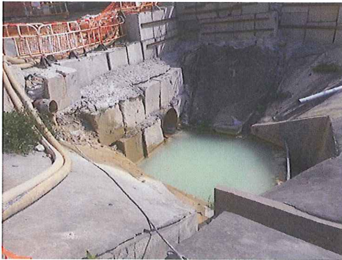
Sand Trap near the grave, treated water discharging.
