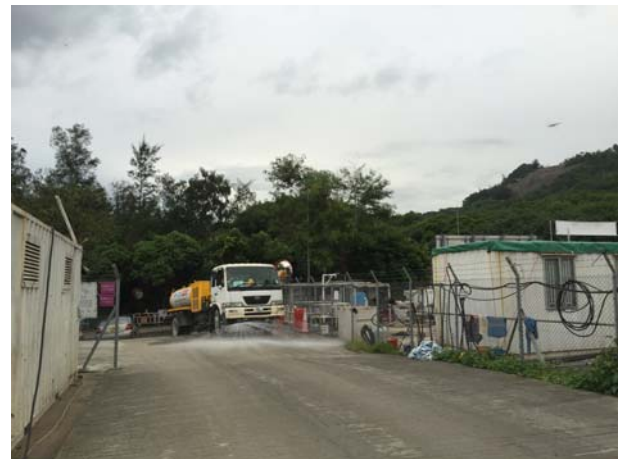
Photo 2 The area of wheel washing bay and site exit was paved with concrete and kept clear of dusty materials
