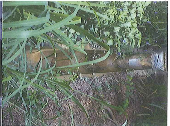
Channel near site office: Treated water discharged and the u-channel need to clear regularly.
