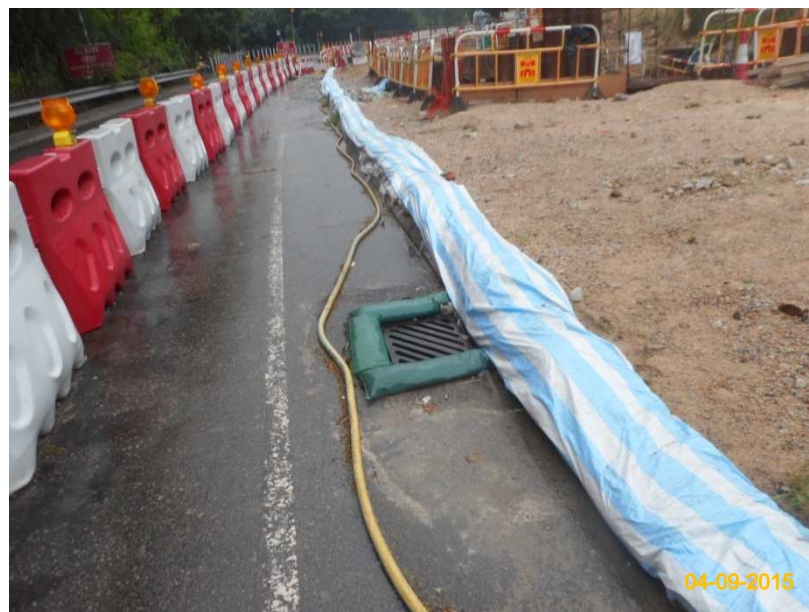
Item 7. Ensure no run-off into water body.
