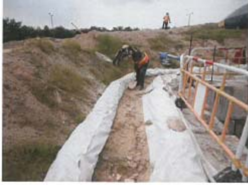
Photo 11: Provide geo-textiles on top of the sandbags located along the top of the cascade's side walls.
