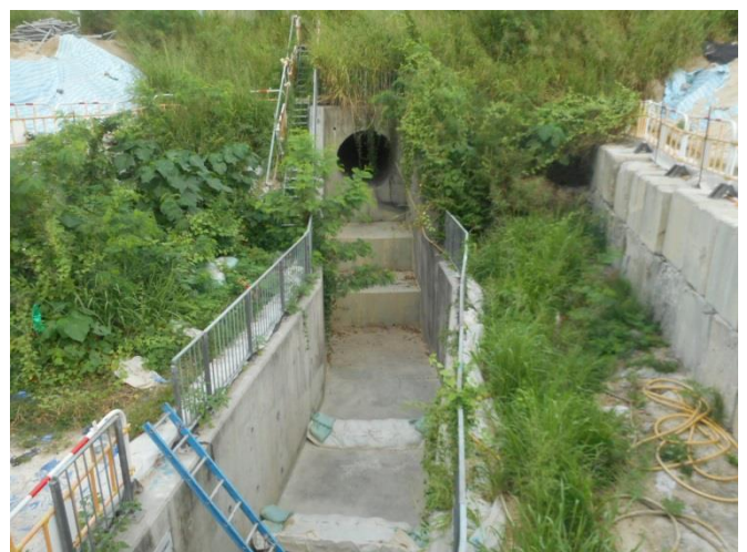
MH5 Cascade: No water is discharging.
