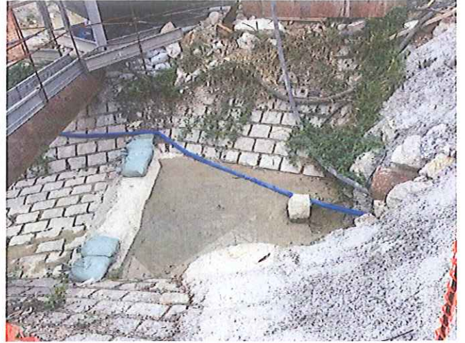
East Portal: Cascade condition
