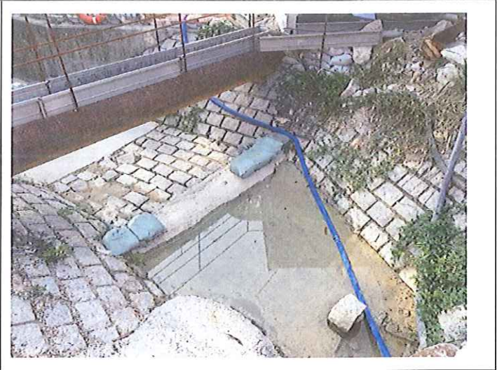
East Portal Cascade condition
