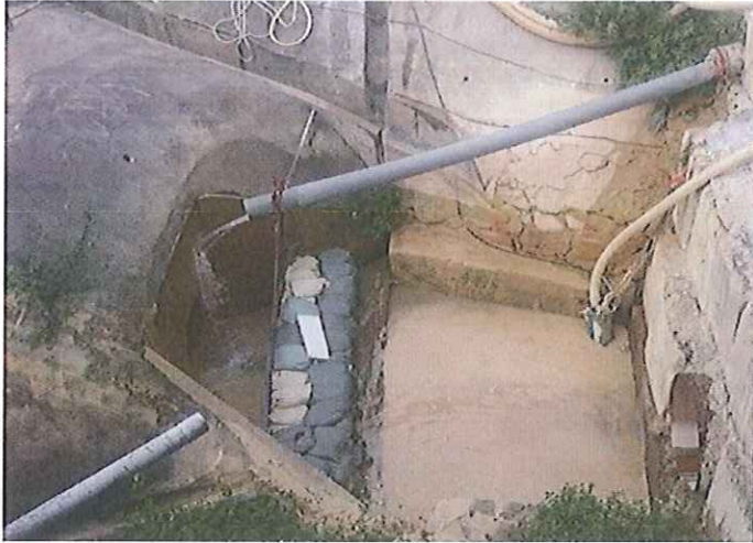
Stream A Outfall: Pumped muddy water to Wetsep and discharging after treatment.
