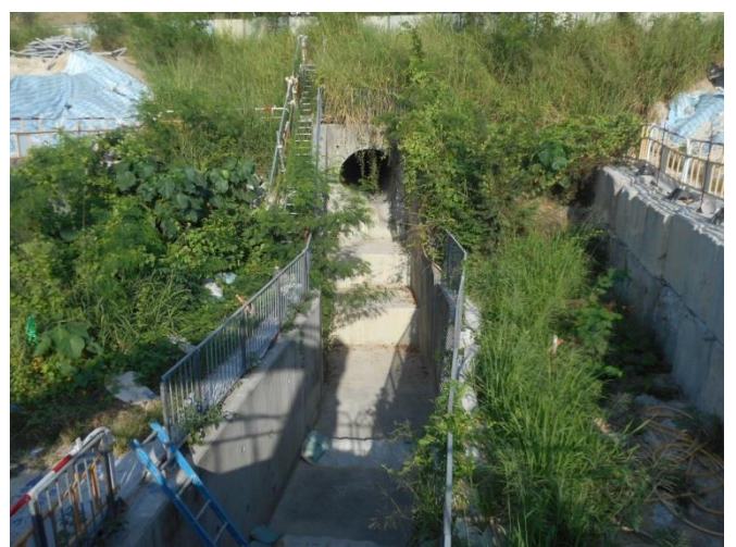
MH5 Cascade: No water is discharging.
