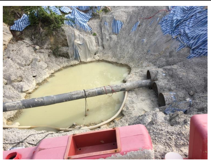
Stream B Pit 1: in normal condition.
