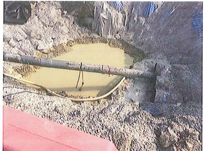
Stream B Pit 1: in normal condition.
