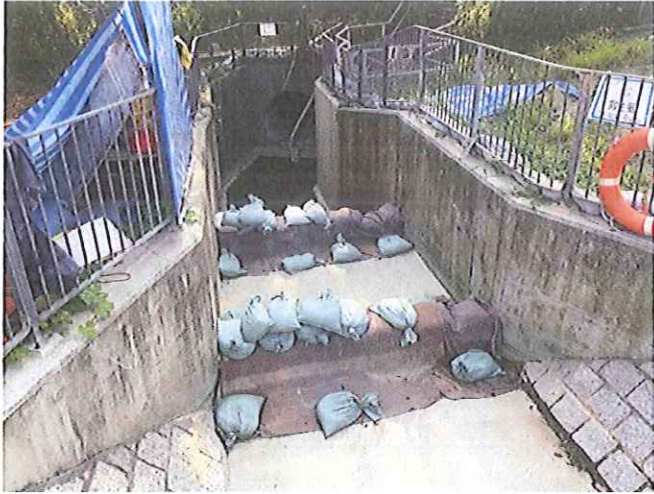
East Portal Cascade: No water is discharged.
