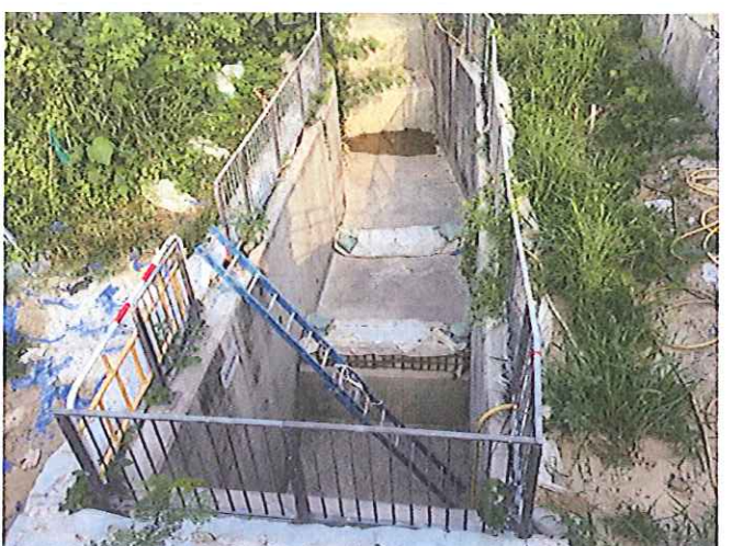
MH5 Cascade: No water is discharging.
