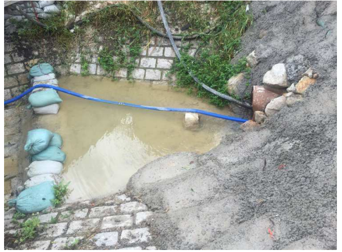
East Portal: Cascade condition
