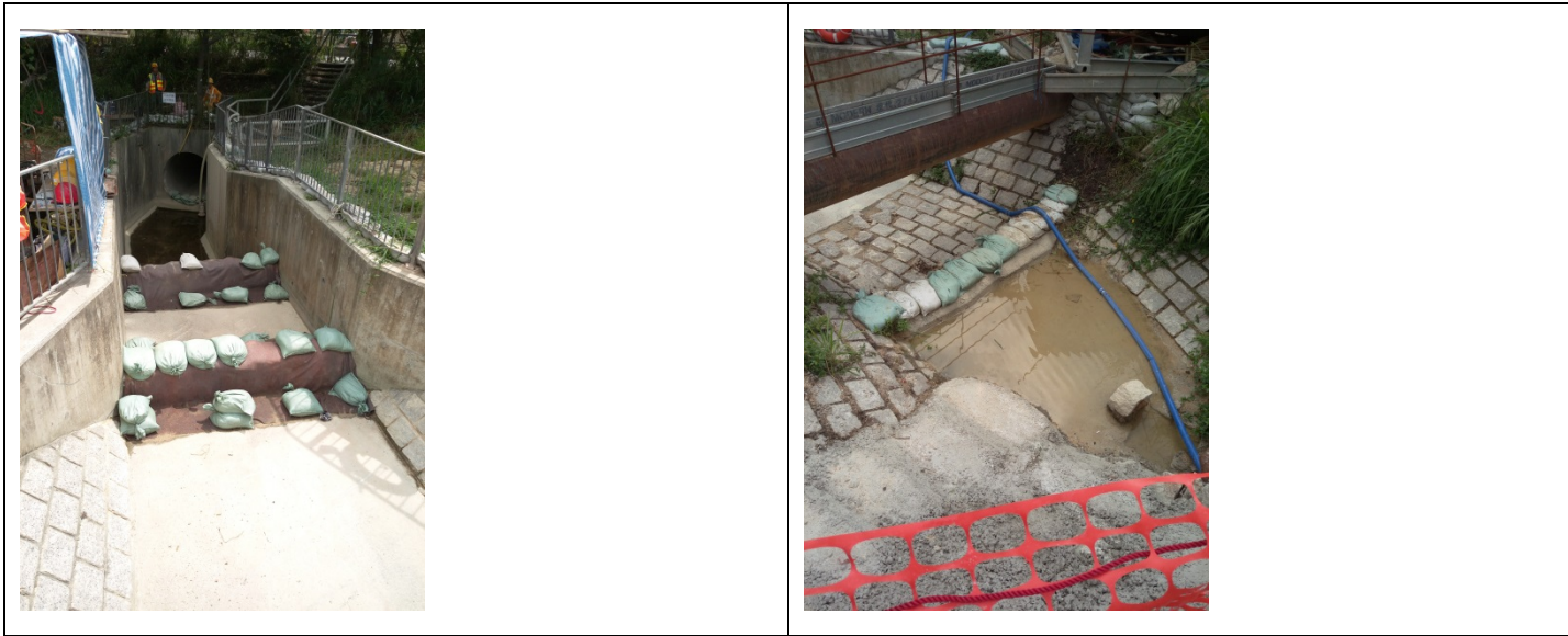
East Portal: Cascade condition
