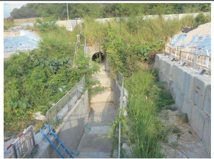
MH5 Cascade: No water is discharging.
