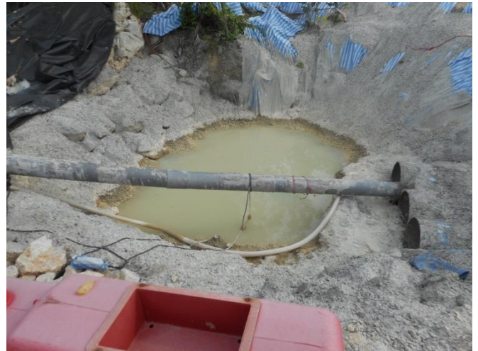
Stream B Pit 1: in normal condition.
