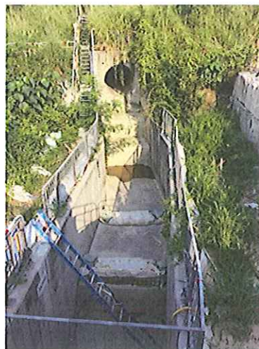
MH5 Cascade: No water is discharging.
