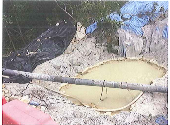
Stream B Pit 1: in normal condition.
