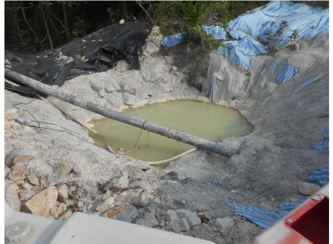
Stream B Pit 1: in normal condition.
