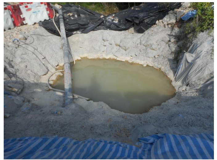
Stream B Pit 1: in normal condition.
