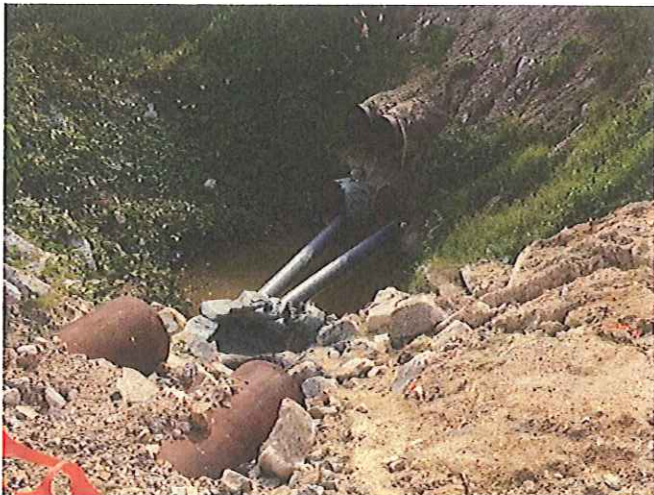
Stream B Pit 2: Treated water was directly discharged to downstream bypass.
