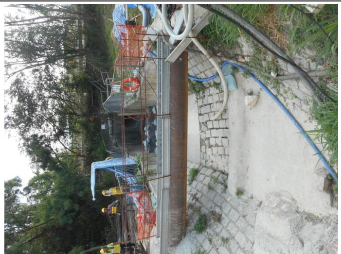
East Portal Cascade: No water is discharged.
