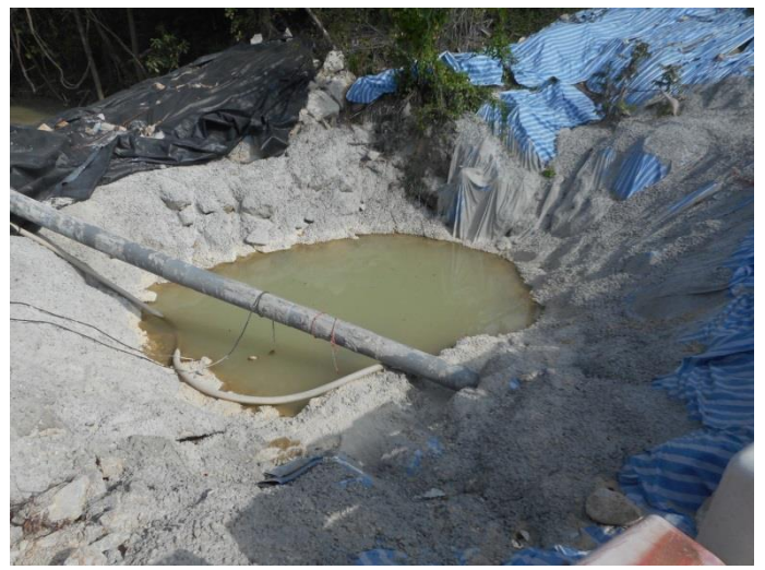
Stream B Pit 1: in normal condition.
