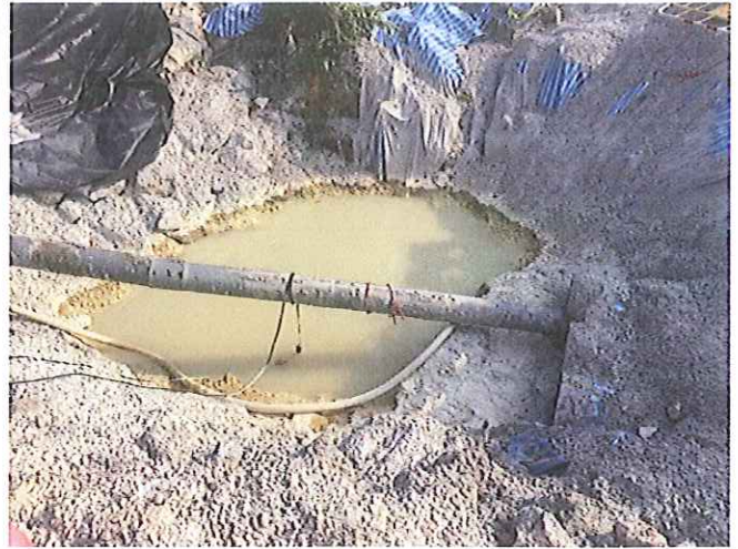
Stream B Pit 1: in normal condition.
