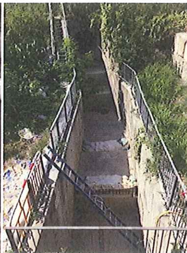
MH5 Cascade: No water is discharging.
