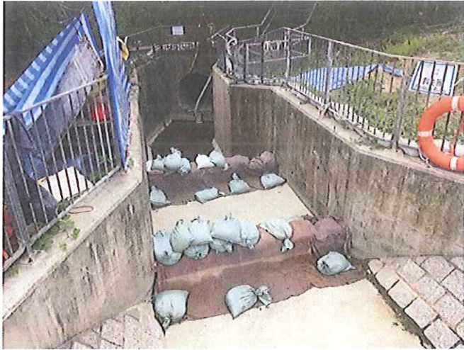
East Portal Cascade: No water is discharged.
