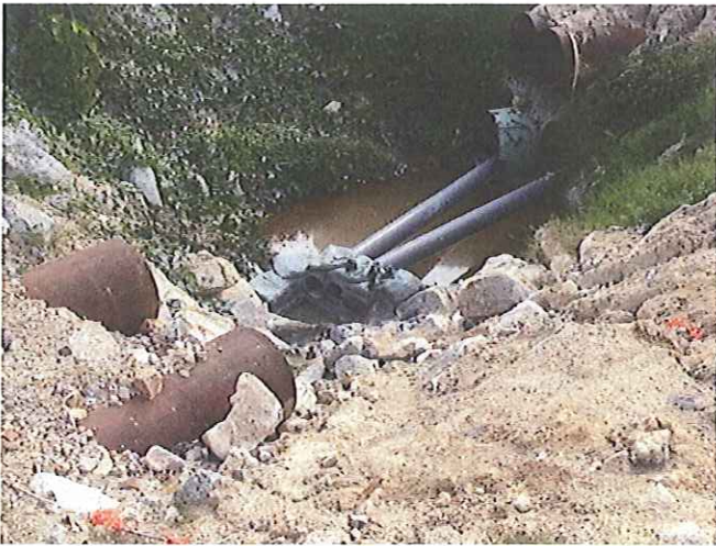
Stream B Pit 2: Treated water was directly discharged to downstream bypass.
