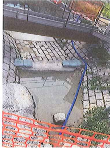
East Portal Cascade condition
