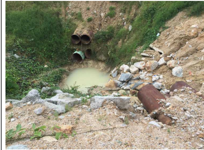
Stream B: Pit 2 in normal condition
