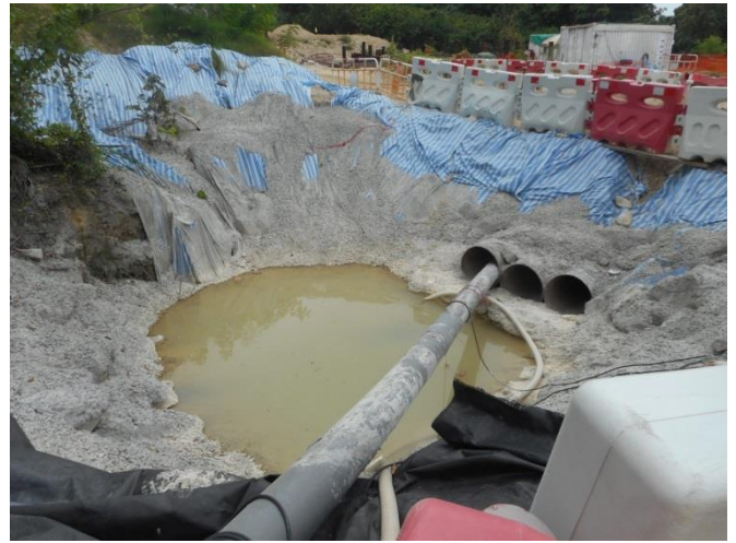
Stream B Pit 1: in normal condition.
