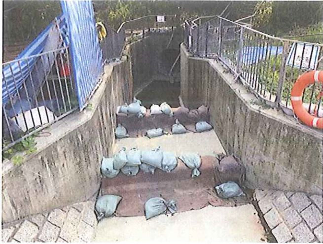
East Portal Cascade: No water is discharged.
