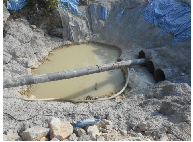
Stream B Pit 1: in normal condition.
