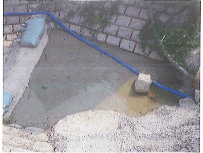
East Portal Cascade condition
