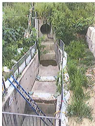
MH5 Cascade: No water is discharging.
