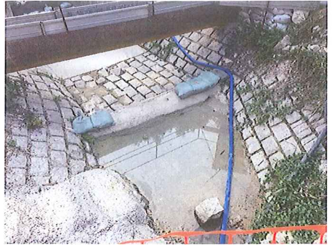
East Portal Cascade condition
