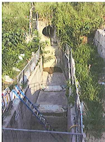
MH5 Cascade: No water is discharging.
