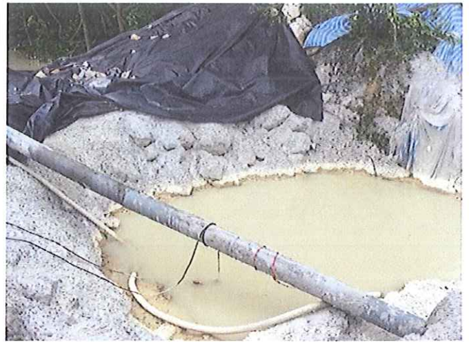
Stream B Pit 1: in normal condition.
