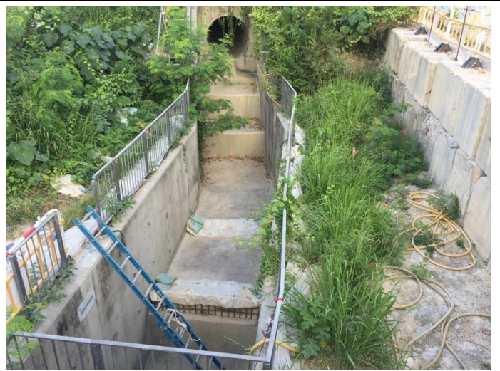
MH5 Cascade: No water is discharging.
