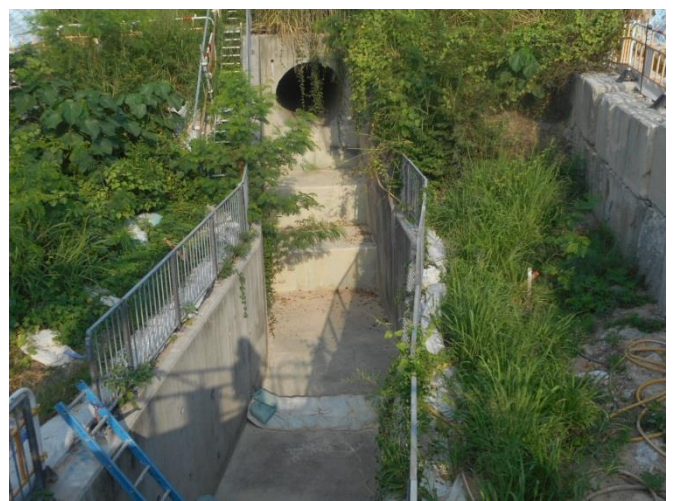
MH5 Cascade: No water is discharging.
