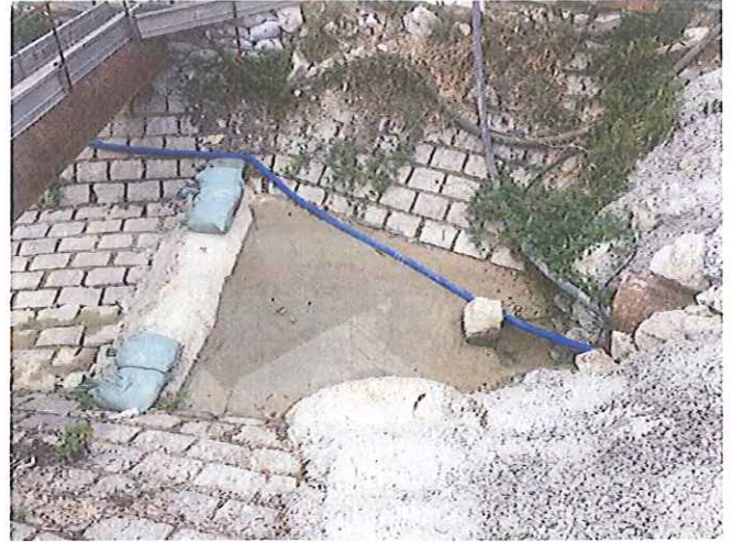
East Portal Cascade condition
