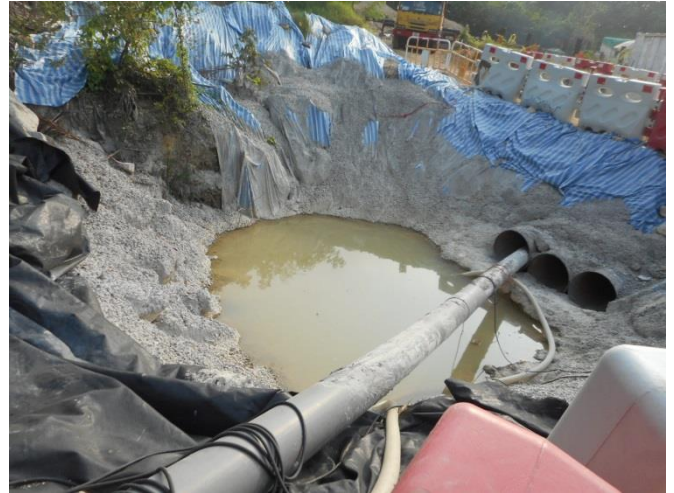
Stream B Pit 1: in normal condition.
