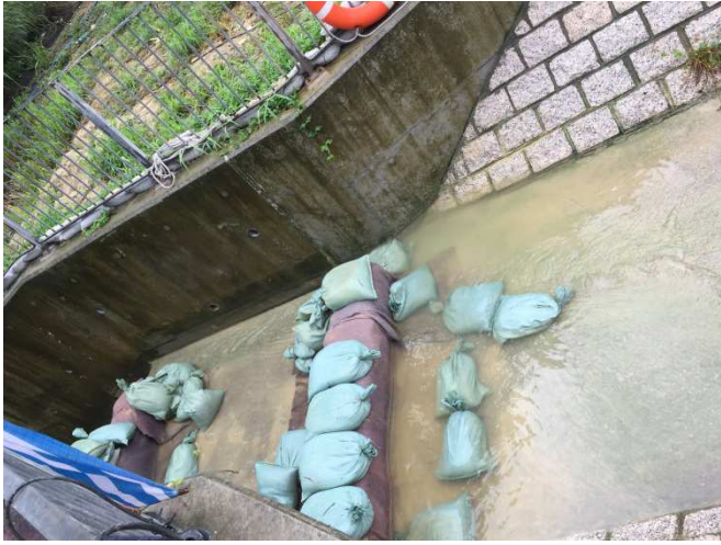
East Portal: Cascade condition
