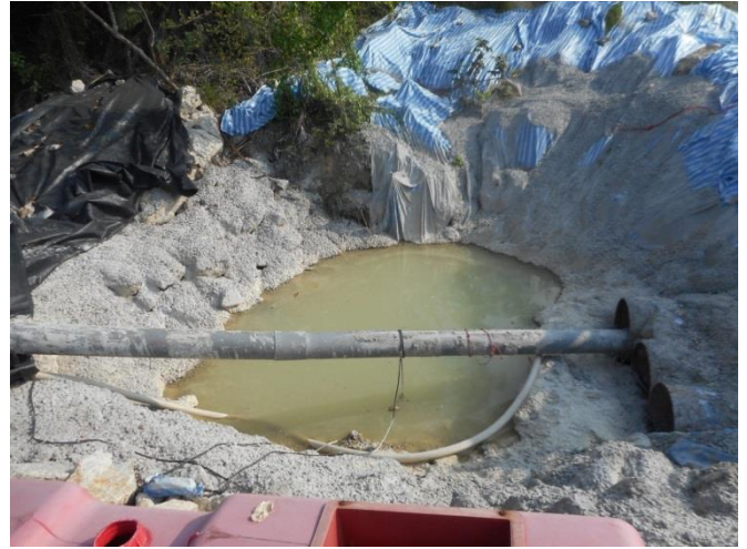
Stream B Pit 1: in normal condition.
