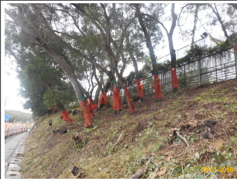
Item 1. Existing trees on boundary of the Project Area have been protected carefully during construction.
