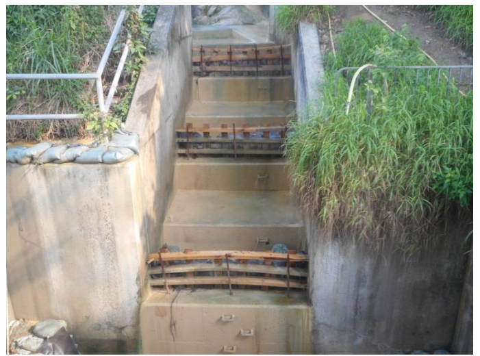
Stream B Outfall: Cascade step channel condition
