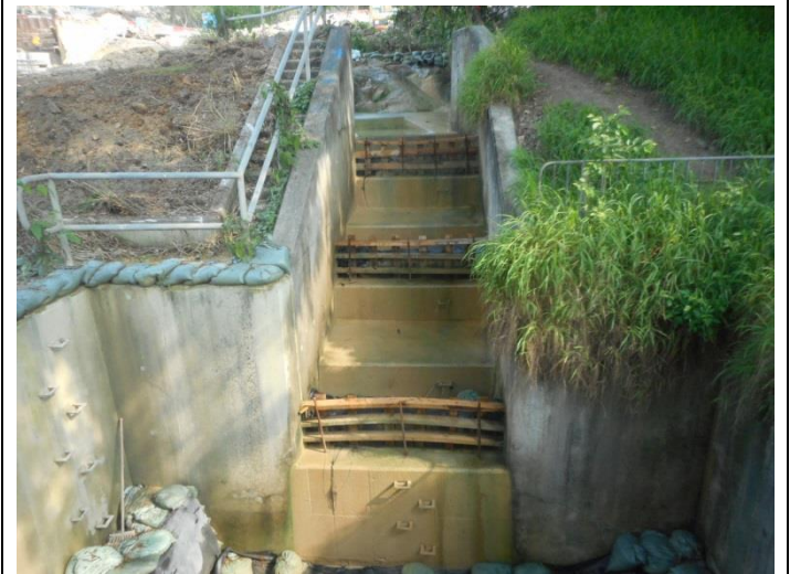
Stream B Outfall: Cascade step channel condition
