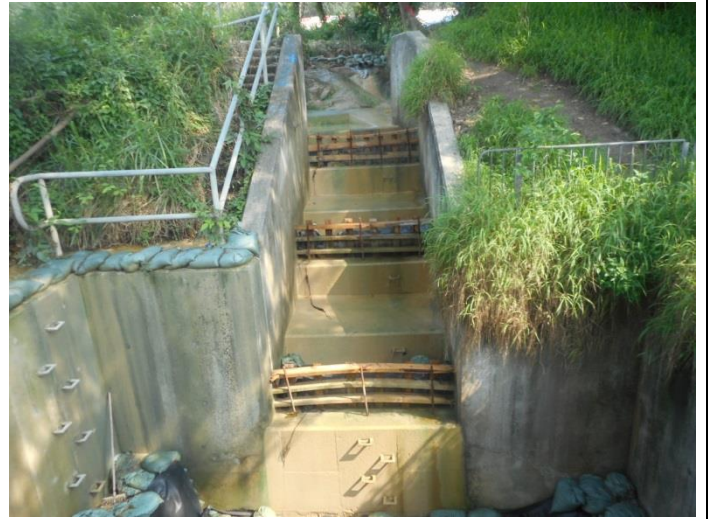
Stream B Outfall: Cascade step channel condition
