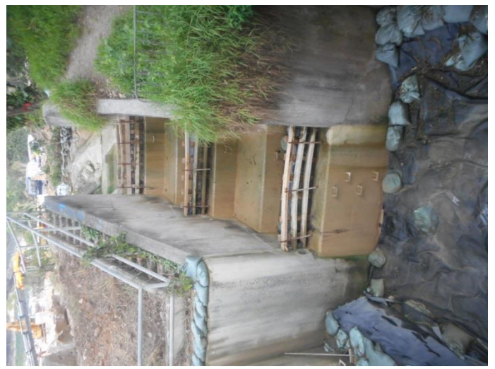
Stream B Outfall: Cascade step channel condition
