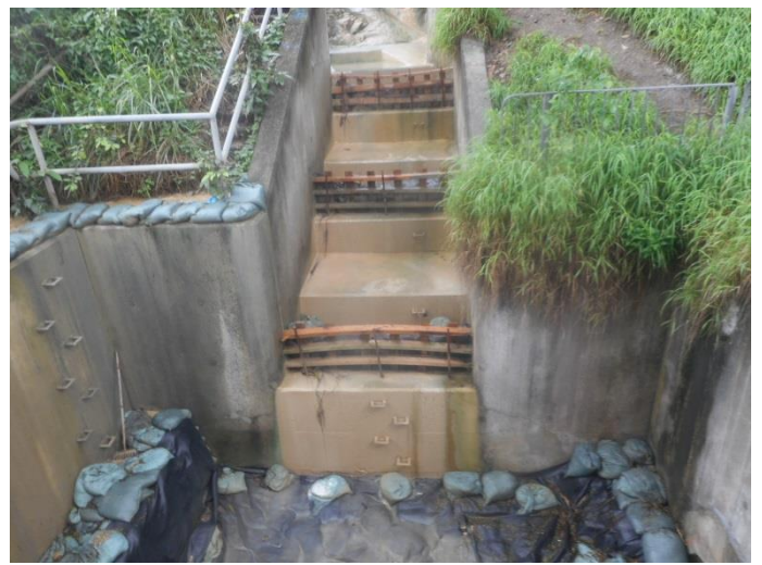
Stream B Outfall: Cascade step channel condition
