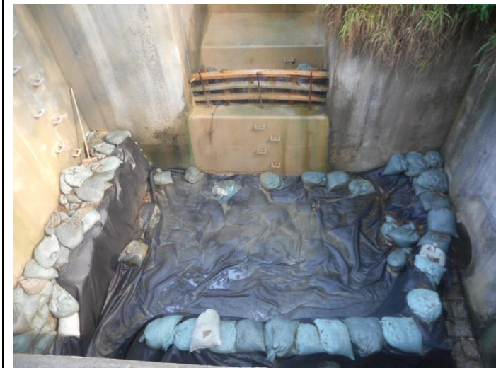
Stream B Outfall: little clean water is discharging.
