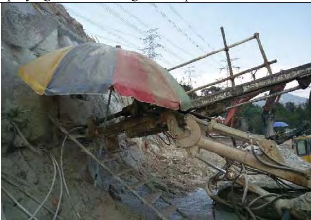
Photo 6 Cover was provided for the “start up” process of the drilling works.
