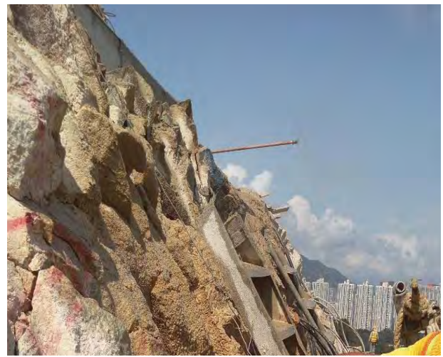
Photo 5 Water sprinkler was provided for the “start up” process of the drilling works.
