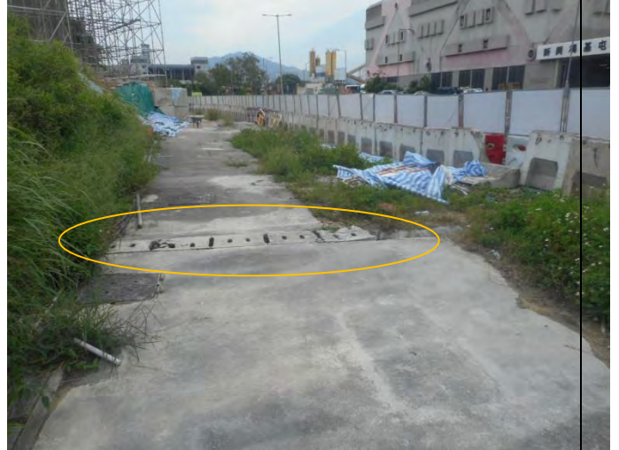
Photo 2 Weekly site inspection on 24 May 2016, no water discharge was observed and the adjacent area of manhole SCH1008705.
