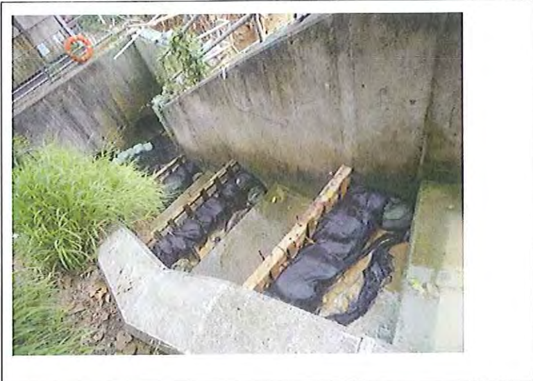
Stream B Outfall: clean water is discharging.
