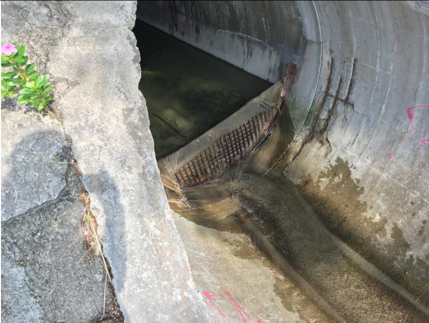
Outfall 1: Clean water is discharging.
