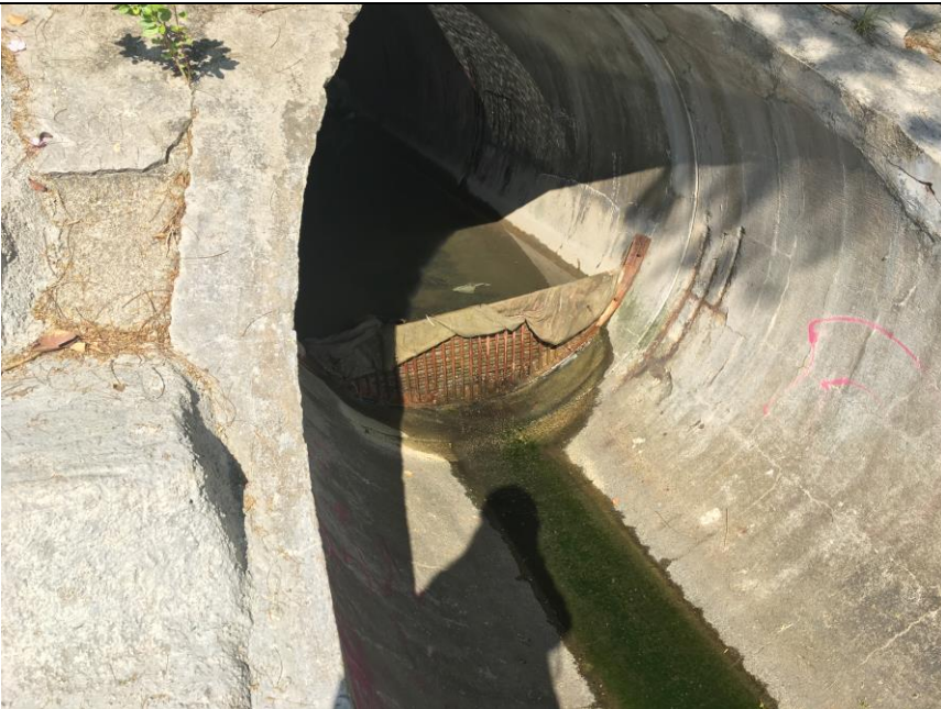
Outfall 1: Clean water is discharging.
