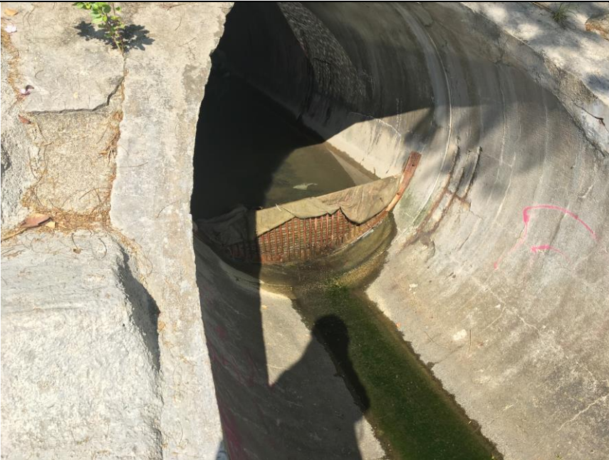
Outfall 1: Clean water is discharging.
