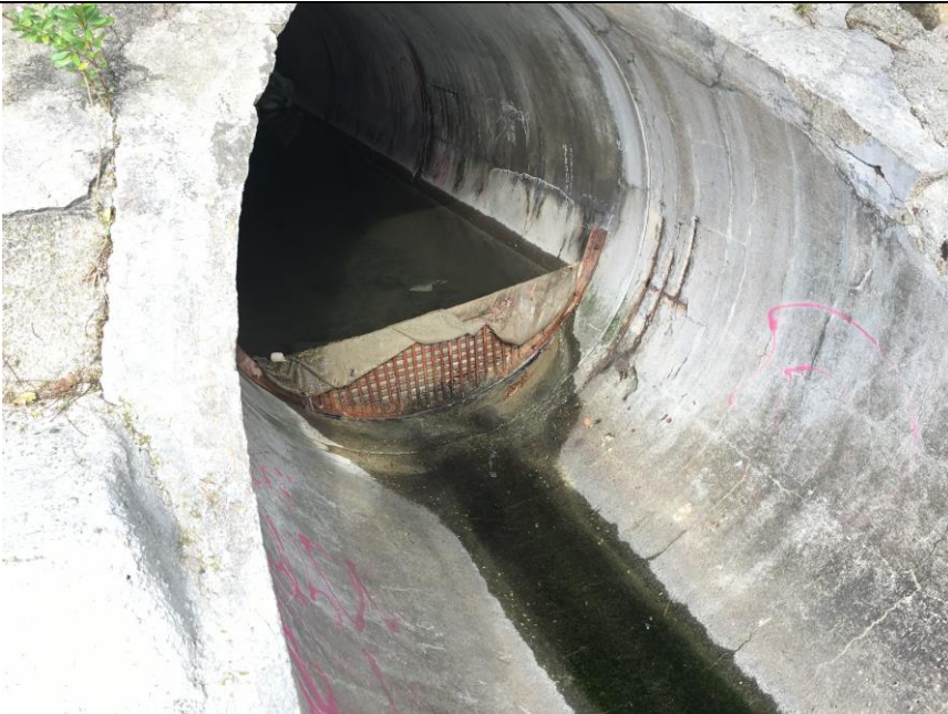
Outfall 1: Clean water is discharging.
