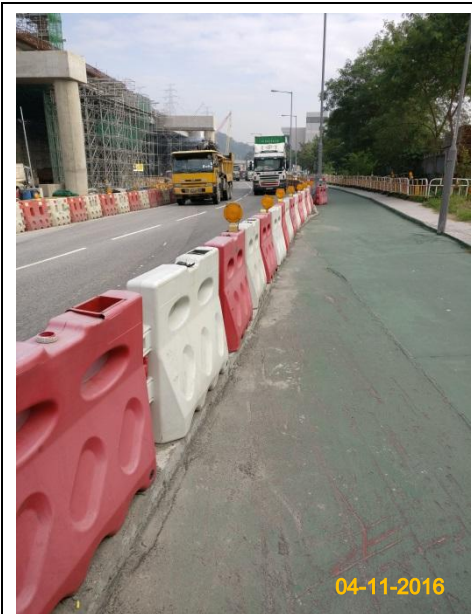
Item 5. Hoarding with panel around works area & Item 6. Temporary traffic management lighting.
