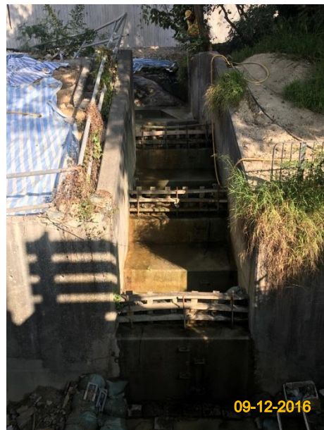
Item 7. Ensure no run-off into water body.
