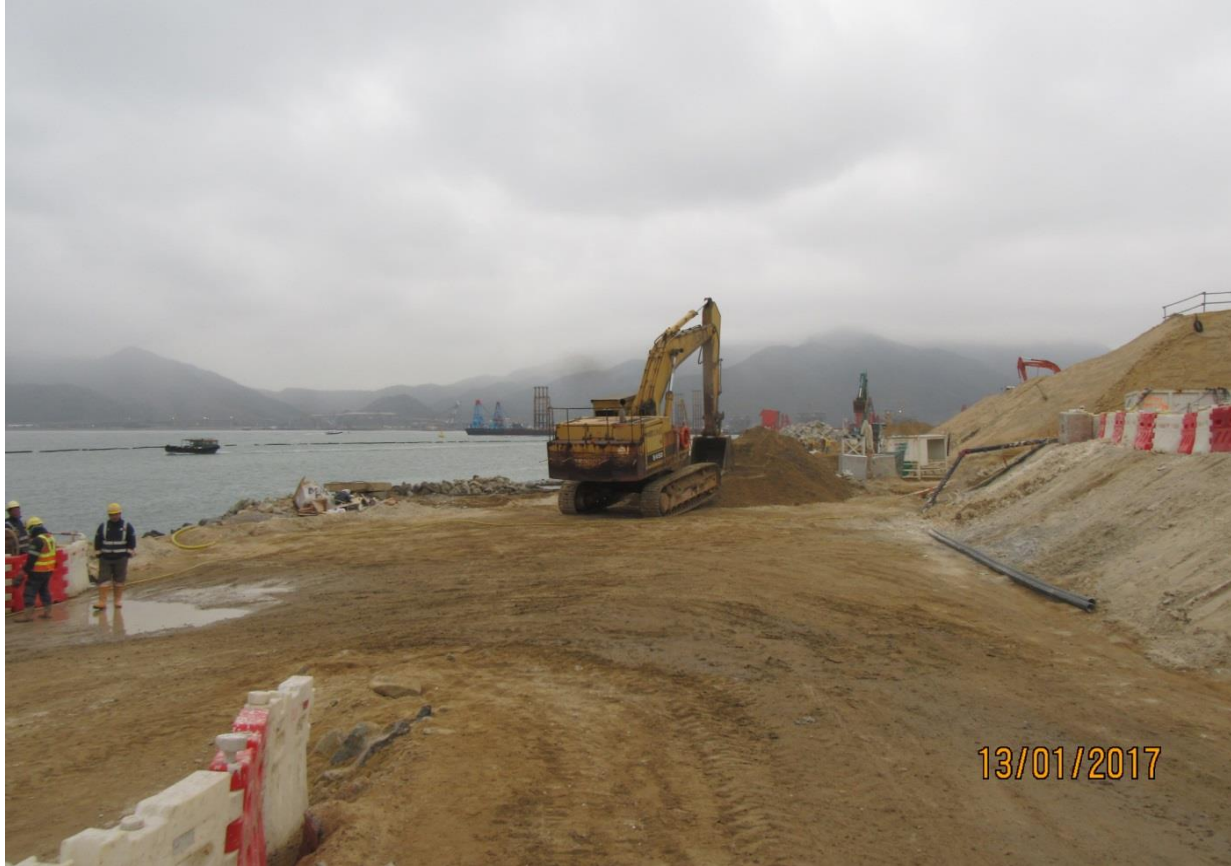
Condition of the site area at the east of HKBCF artificial island which did not reveal any observable evidence of improper discharge
