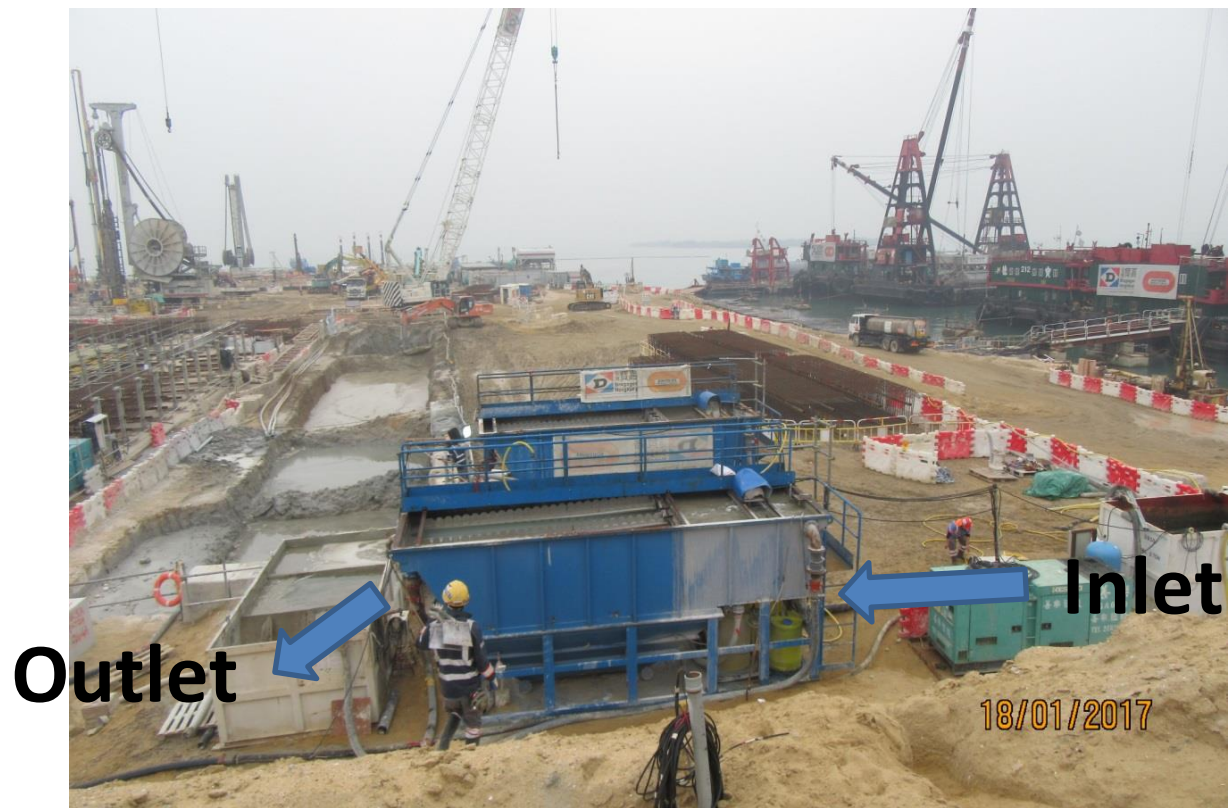
Wastewater was treated in the Wetsep before discharge.
