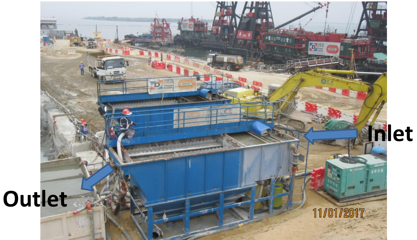
Wastewater was treated in the Wetsep before discharge.
