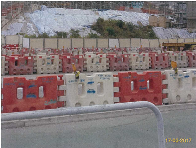
Item 5. Hoarding with panel around works area & Item 6. Temporary traffic management lighting.
