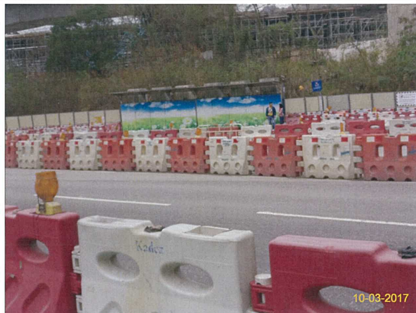
Item 5. Hoarding with panel around works area & Item 6. Temporary traffic management lighting.
